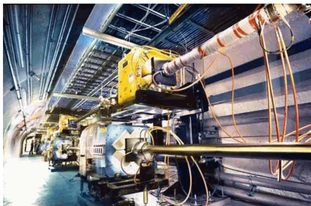
Figure 1 View of the PEP-II tunnel.
