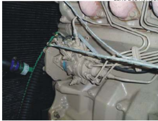
Figure 13. Diesel fuel pump and governor.
