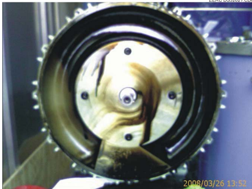
Figure 34. Tar condensation in the process blower.
