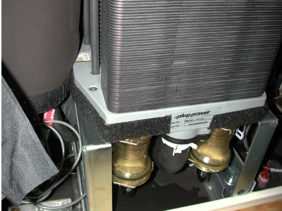
Fig. 21. Photograph of the inside, left-hand (as you look at it) corner of the GenCore unit. There is a colorless liquid present on the bottom of the unit; most likely this is ethylene glycol-based coolant.
