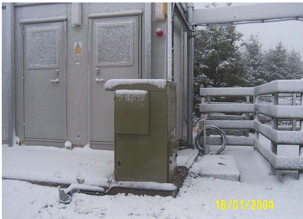
Figure 16: GC5T Installed and Operational at a Site Host's Telecommunications Facility
