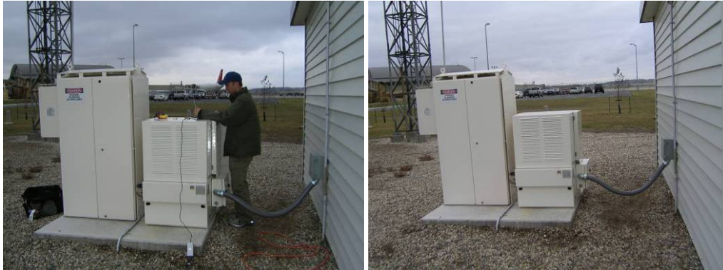
Figure 20: Commissioning of the FAA unit
