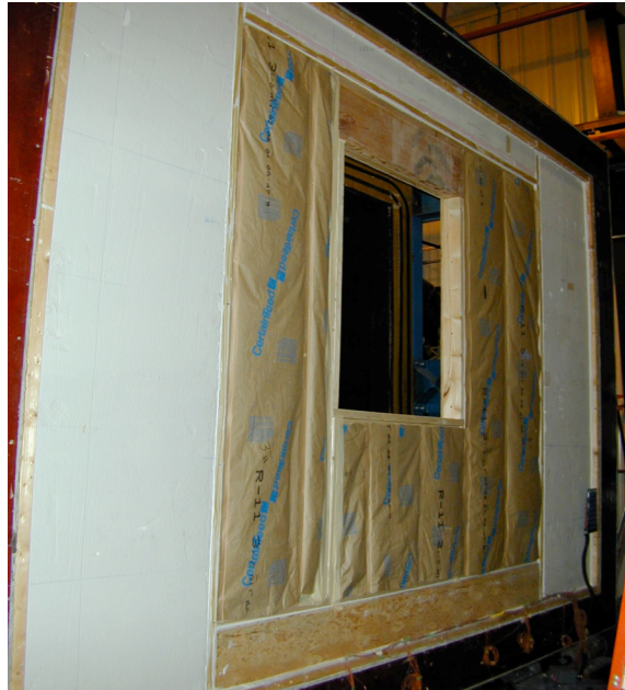
Figure 4. Wall frame after insulation placed in cavity and RGHB guard insulation added
