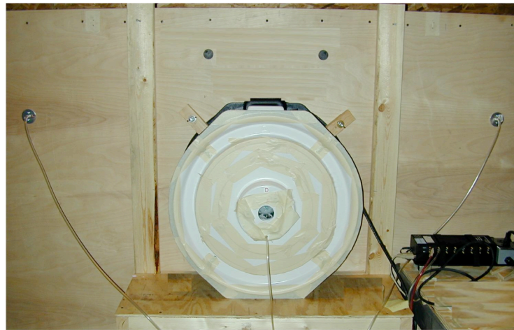
Figure 12. Panel to Adapt Blower Door Fan to Enclosure over Retrofit Base Wall
