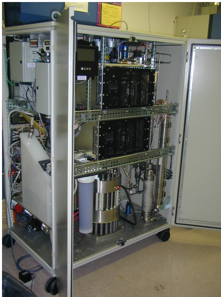
Figure 10. 2000-psig (13.9 MPa) Electrolyzer System (EP-2)
