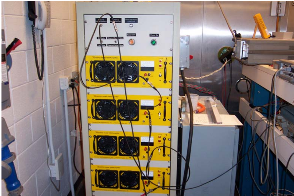
Fig. 2.2. Current amplifier rack.
