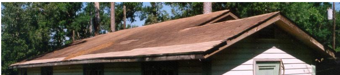
Figure 3.3. House with a roof in need of replacement.
