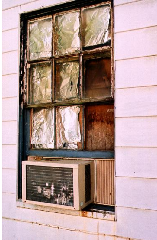
Figure 3.5. Weather damaged window in need of replacement.
