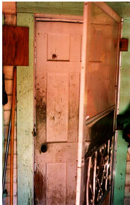
Figure 3.6. Door in need of replacement.
