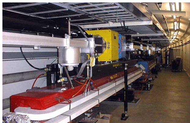
Figure 1. Tunnel layout of the two beam lines. The LER is above the HER.
