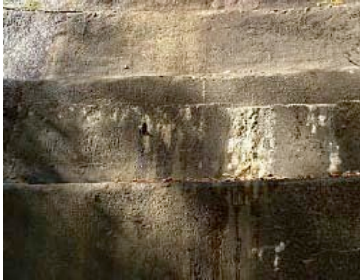
Figure 4.10 Efflorescence in water structure.
