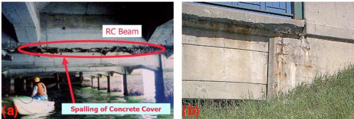
Figure 4.24 Corrosion of reinforced concrete: (a) sea water structure, (b) bridge structure.
