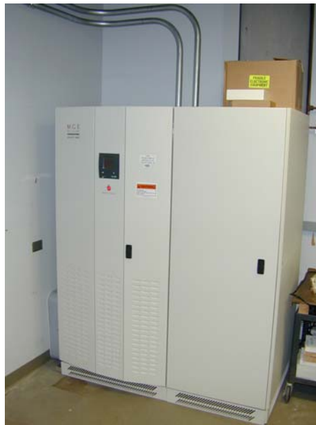
Figure 10. Installed Back-Up Power Supply System for Gradient Test Systems
