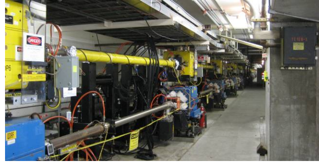
Figure 3. LER vacuum chamber in IR12 (upper beam pipe). The outer clearing solenoid can be seen.
