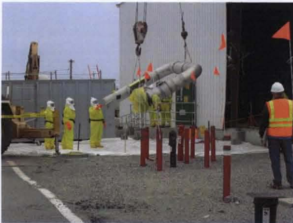
Removing 241-Z Exhaust Duct from Building to Load in to Special Transport Container
