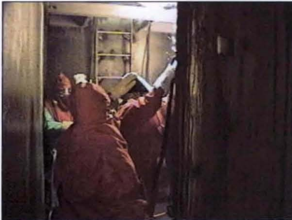
Using Plasma Arc Torch to Cut Access Opening in 241-Z Waste Tank
