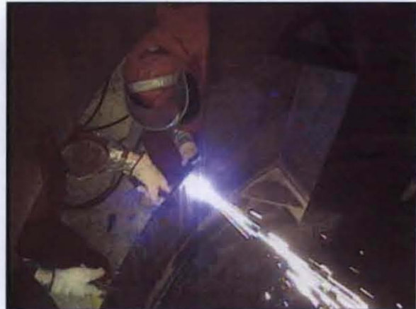
Using Plasma Arc Torch to Cut Access Opening in 241-Z Waste Tank
