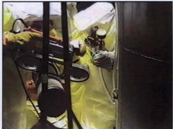
Size Reducing Process Pipe on the Tank Vault Floor
