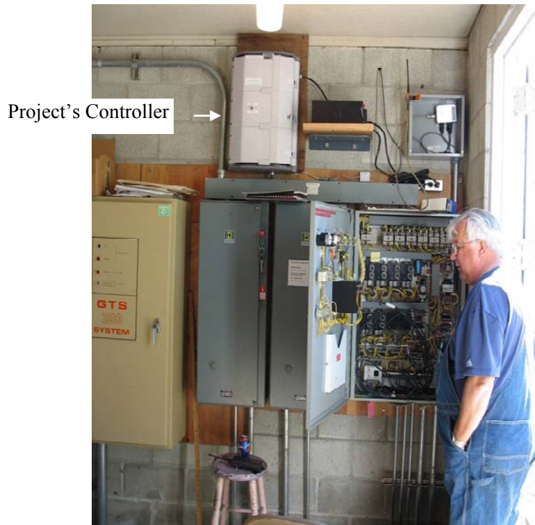
Figure 5.4. Control Panels at the Sekiu Pumping Station
