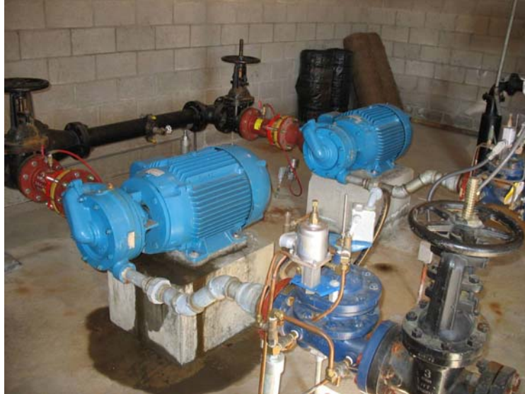
Figure 5.1. Pumps at the Sekiu Water Pumping Station
