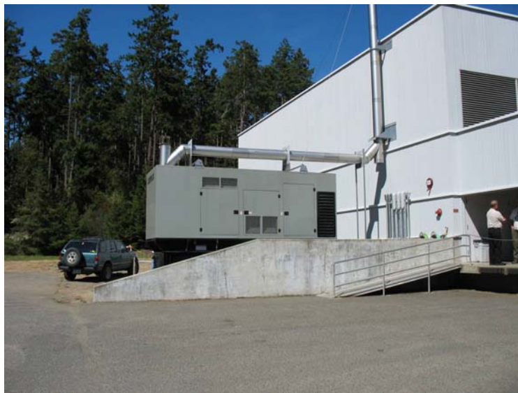
Figure 6.1. PNNL's 600-kW Caterpillar Diesel Generator in Sequim, Washington
