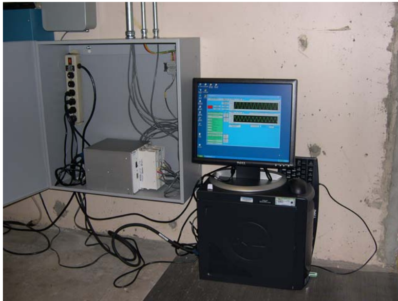
Figure 9 PPSM Monitoring Unit at BPA's Portland Headquarters
