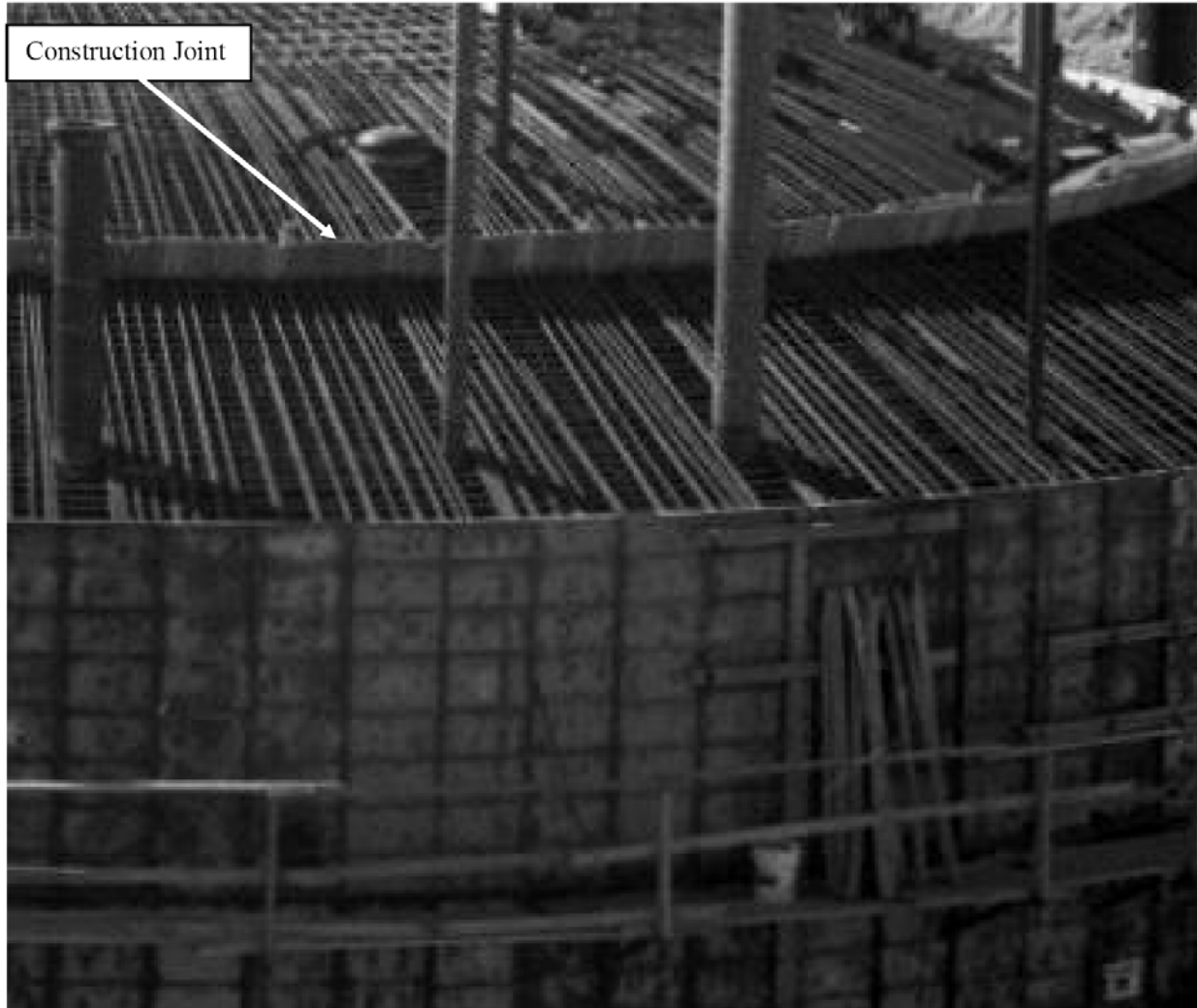
Figure 6. Example of Concrete Construction of the Tank Dome Showing the Location of the Construction Joint, 241-SY Tank Farm
