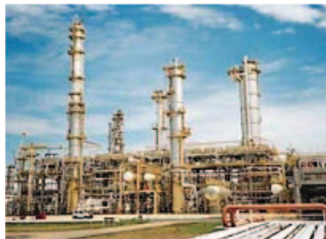
Fluid heating in a petroleum process heater.
