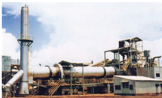
A rotary dryer for removal of free water.
