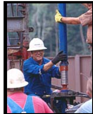
Figure 4-6. Multi-stage electrical submersible pump used for testing and sampling a deep brine reservoir (Photo courtesy of Seah Nance, Texas Econ. Bur. of Geology).
