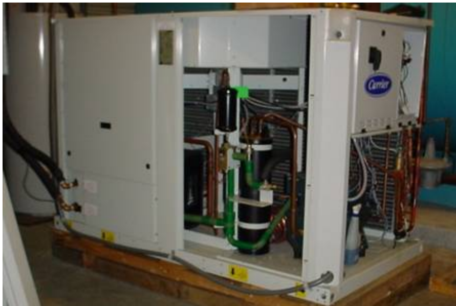
Figure 7.5: Installation at Druid County Hospital
