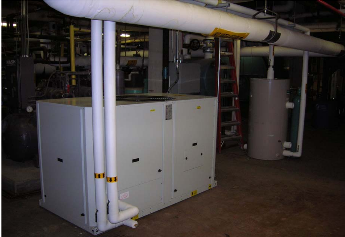
Figure 11.4: Mechanical room installation at Eastern Health Services
