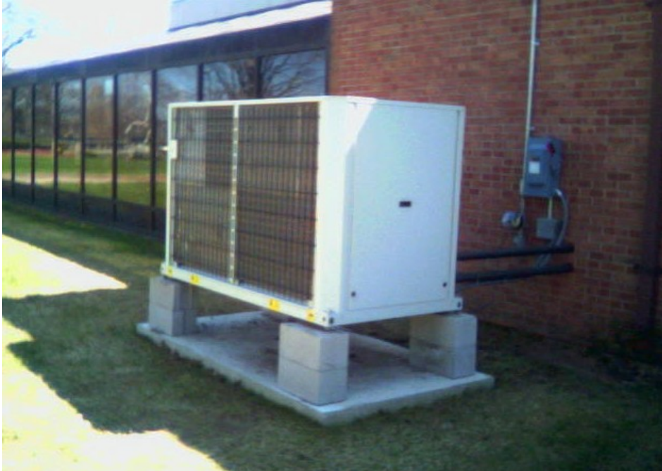
Figure 7.4: UTRC cafeteria outside installation
