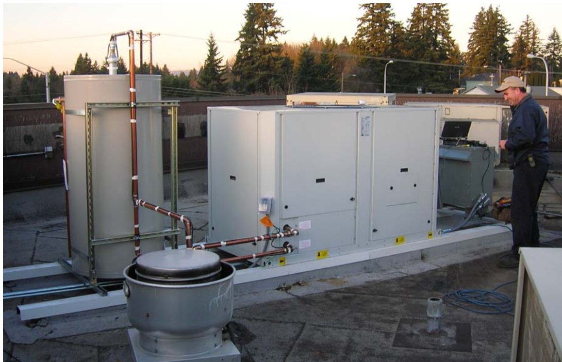
Figure 11.5: Rooftop installation at Shari's Restaurant in Portland Oregon
