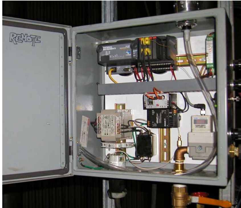
Figure 4.31. Picture of Probe 5 box and instrumentation.
