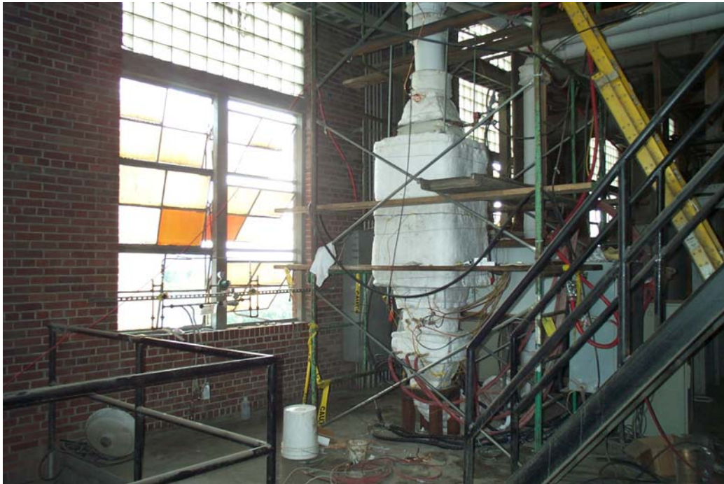
Figure 5.94. Slipstream reactor after insulation.
