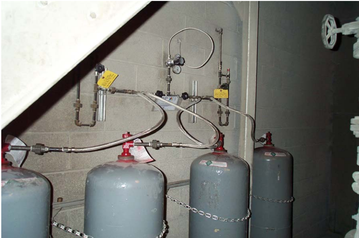
Figure 5.77. Four 150-lb ammonia cylinders connected to the ammonia supply manifold in the Unit 1 Fan room.
