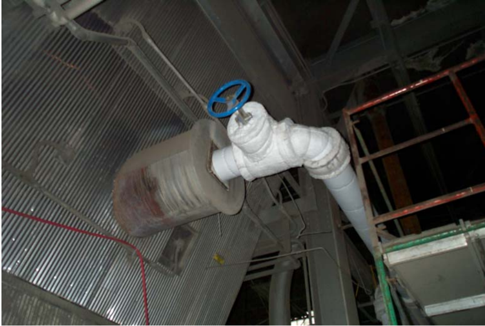
Figure 5.97. Outlet port located downstream of air heater.
