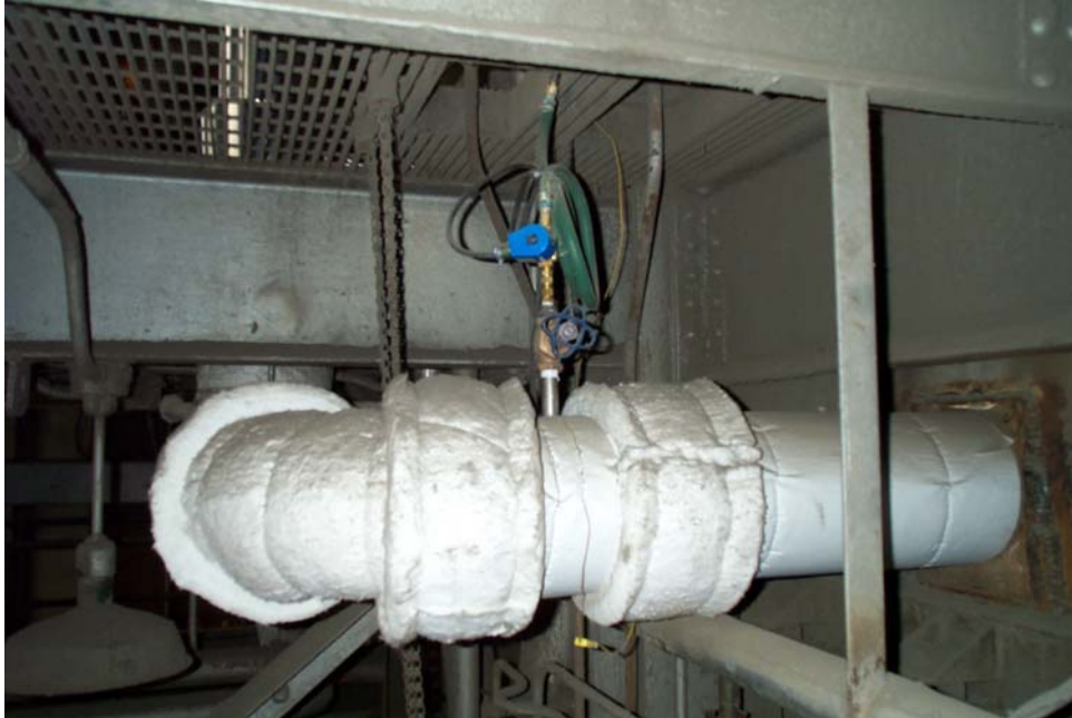
Figure 5.96. Inlet port located upstream of air heater.
