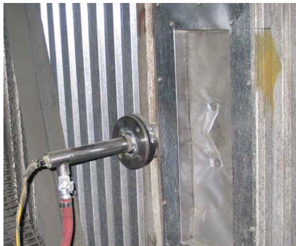
Figure 4.35. Main corrosion probe installed at Gavin Unit 1. Cutout at right was for access to passive probes installed adjacent to electrochemical probe.
