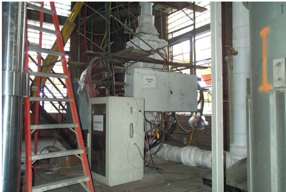
Figure 5.95. Control Box and Sequencer.
