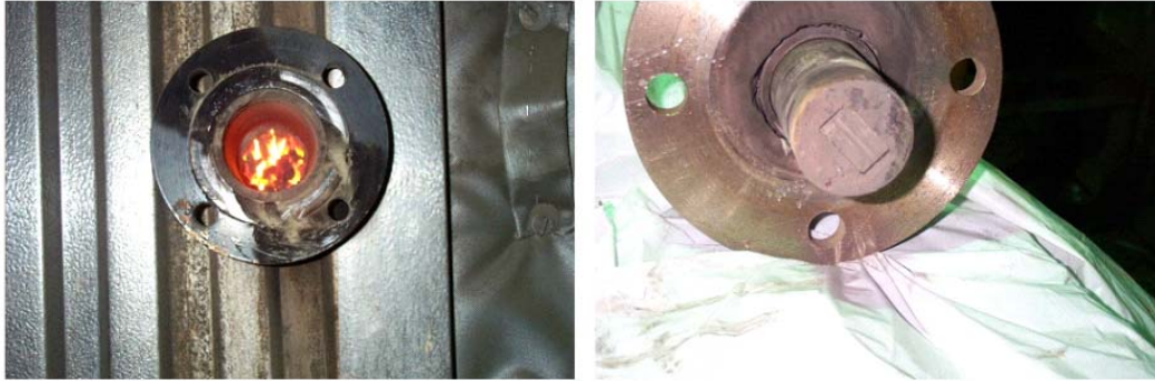
Figure 4.36. Corrosion probe boiler access port and probe after operation in boiler.
