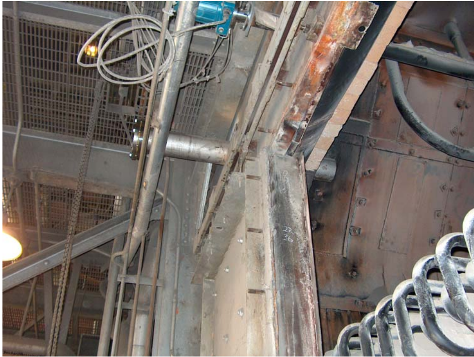
Figure 5.91. Inlet port installed at economizer exit at Plant Gadsden.
