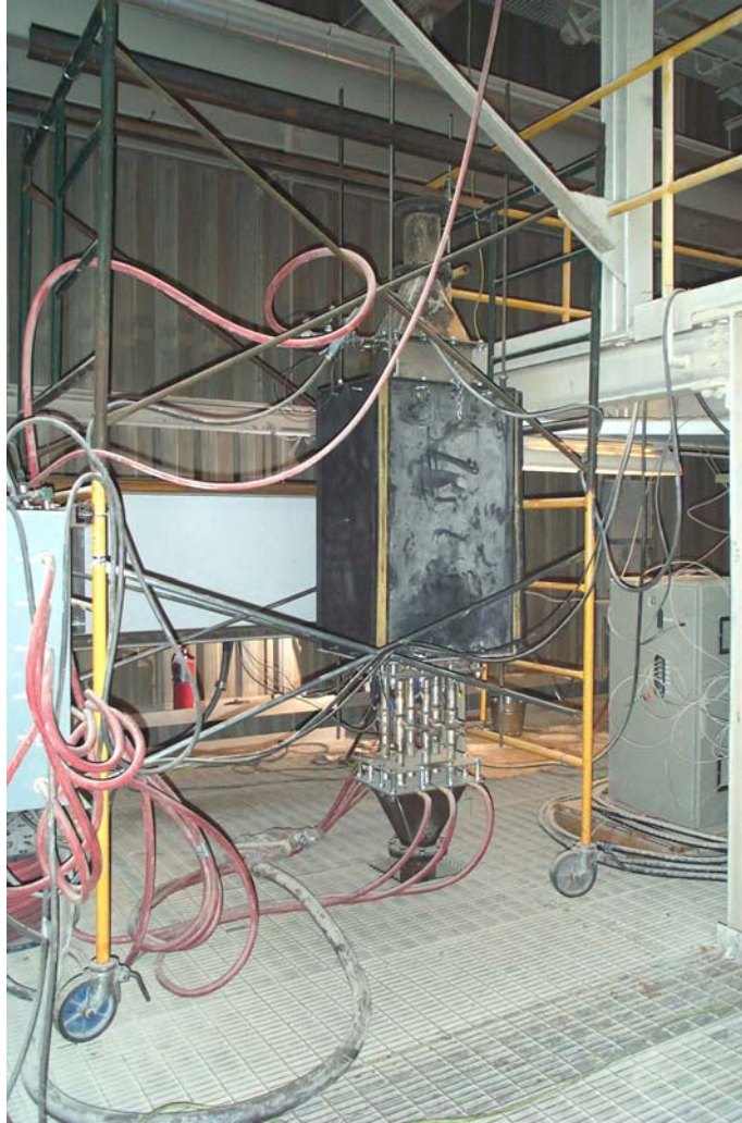
Figure 5.74. SCR Unit installed between the economizer and the air heater at Rockport Plant.
