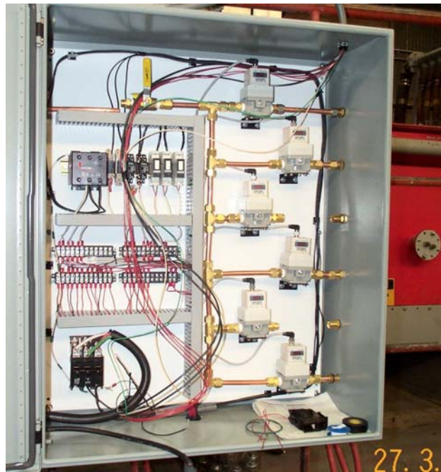
Figure 5.71. Electronics box for the slipstream reactor.
