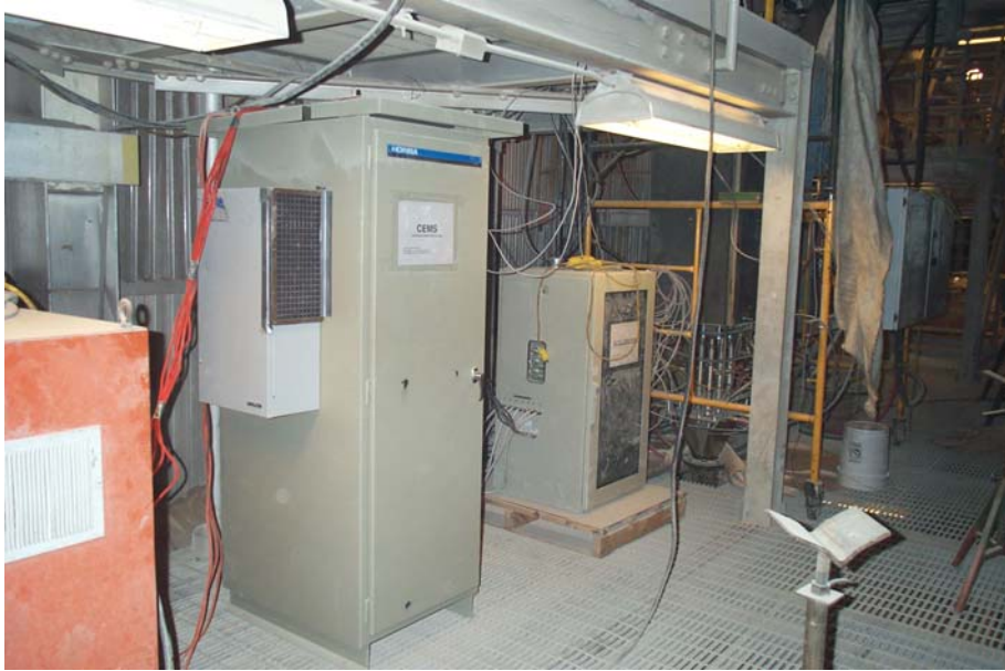
Figure 5.75. CEMS and SEQUENCER cabinets installed at Rockport Plant.
