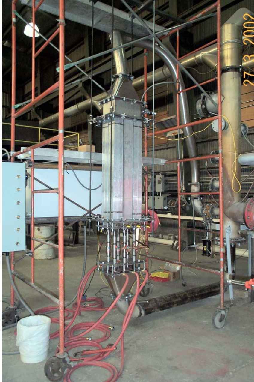
Figure 5.69. Multi-catalyst slipstream reactor with outer doors removed to show catalyst chambers.
