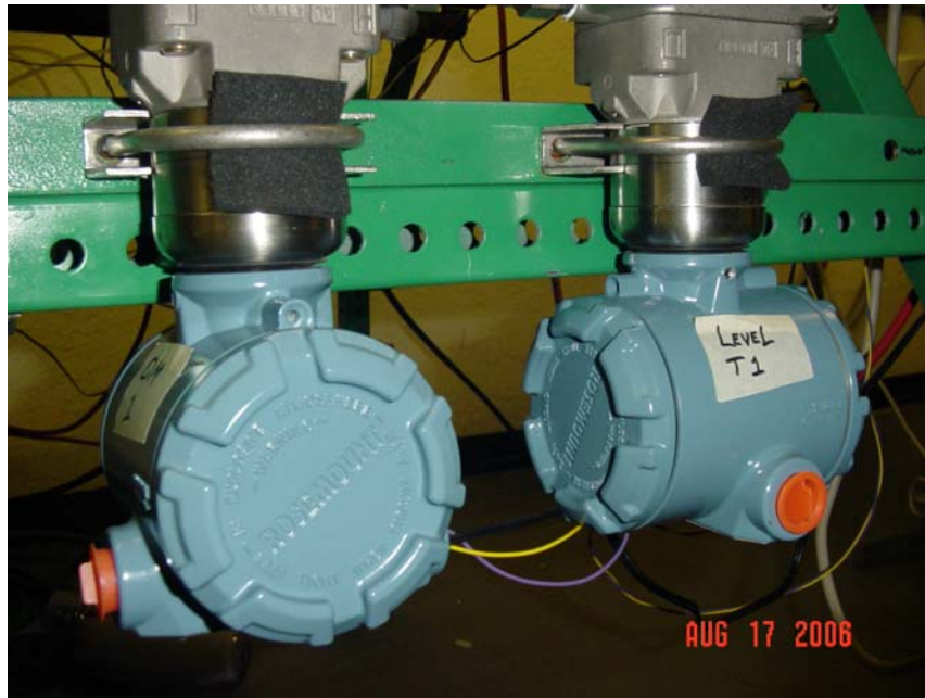
Figure 6.6. Pressure sensors used in the loop.
