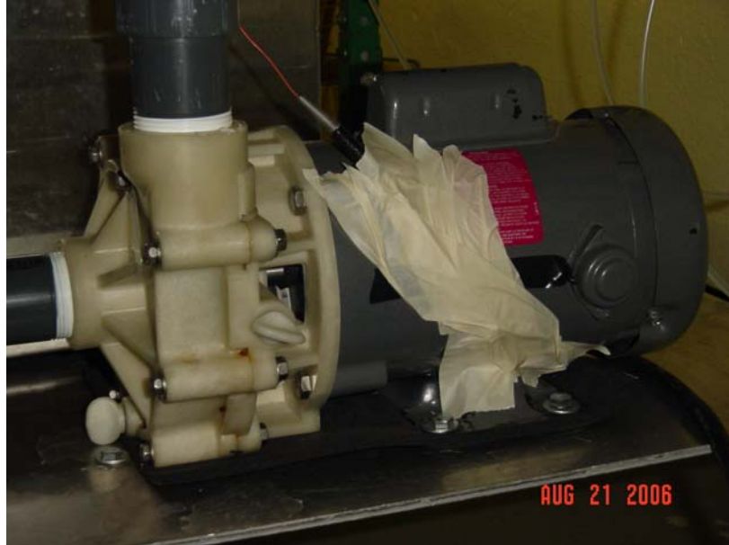
Figure 6.11. Centrifugal pump and thermocouple.
