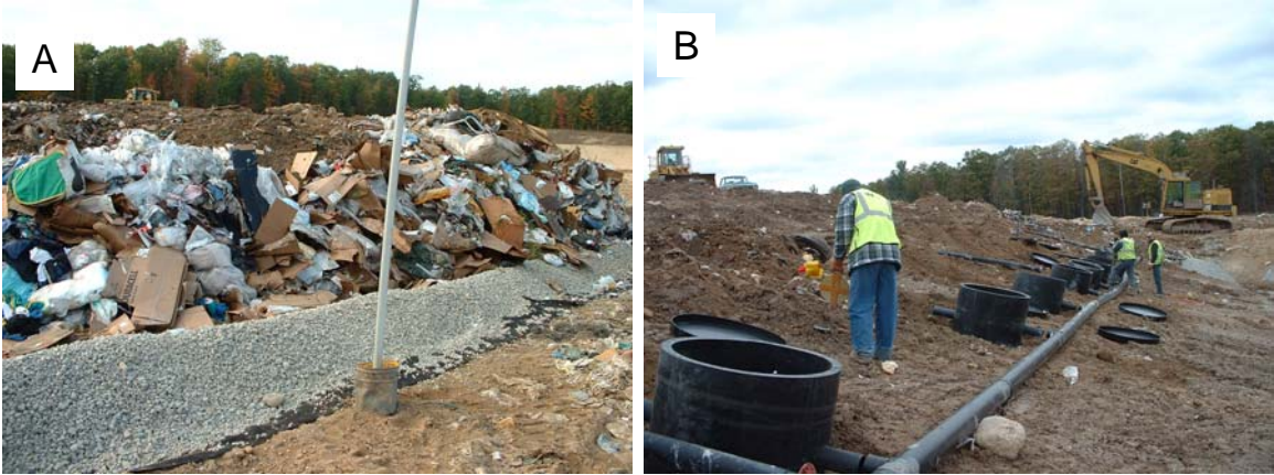
Figure 4-8: Gas extraction line (A) and gas collection manifold (B)
