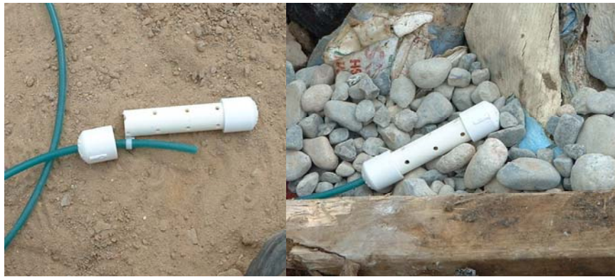
Figure 3-9: Gas sampling port
