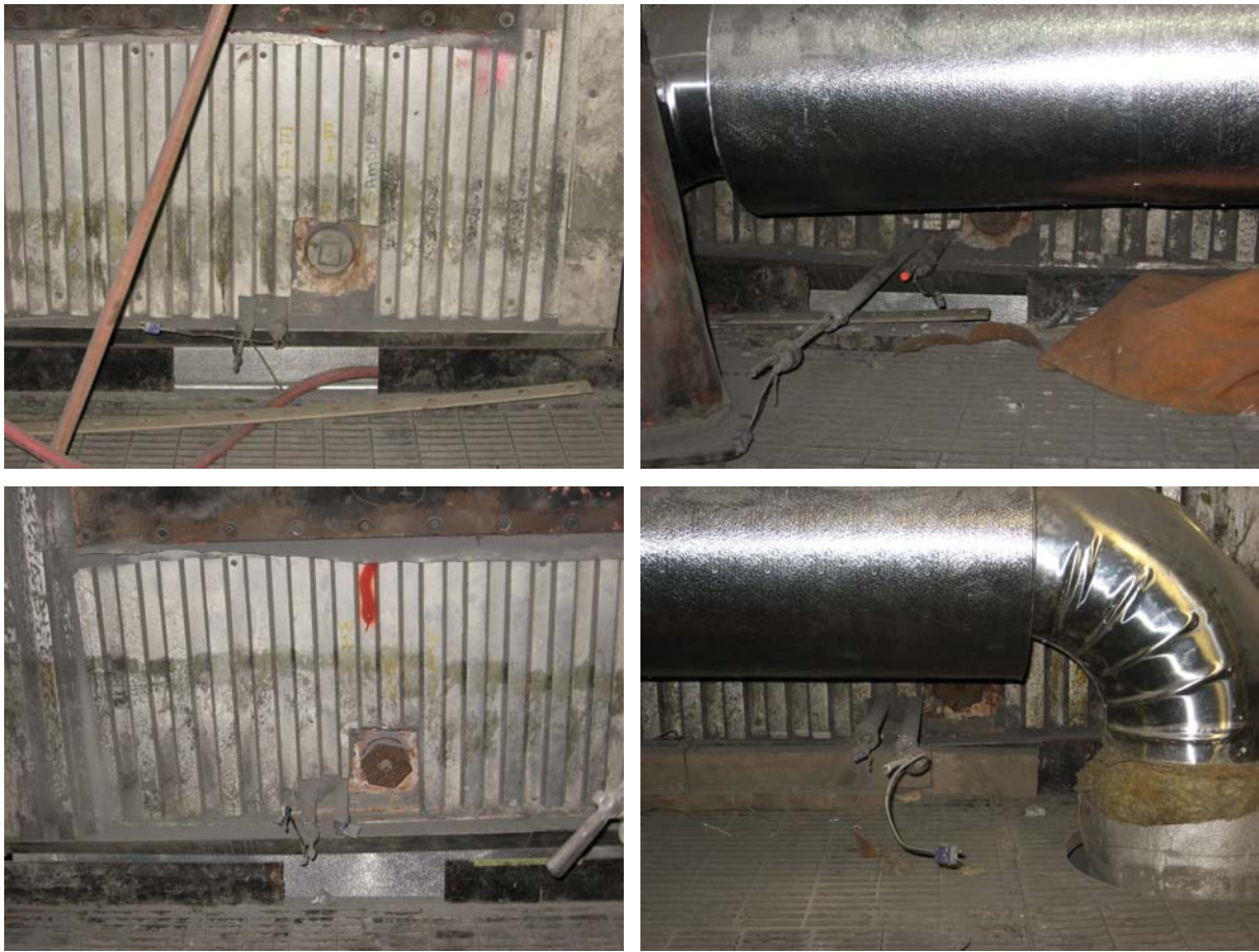
Figure 2. Economizer outlet sampling ports
