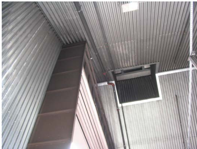
Figure 2-7 The top-north corner of the large door in the 'up' position
