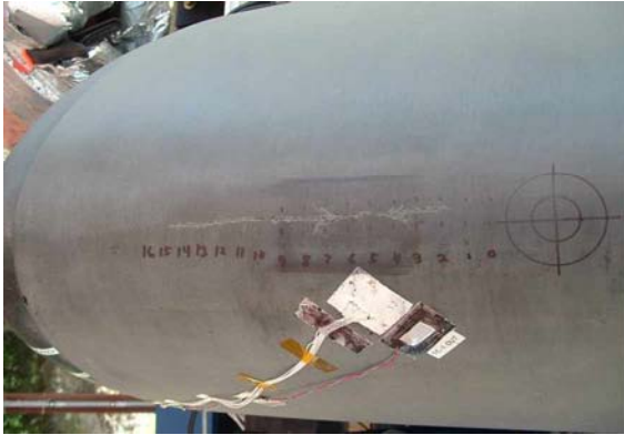
Photo of Crack at Apex
