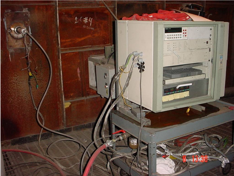
Figure 16. Power plant waterwall measurement.
