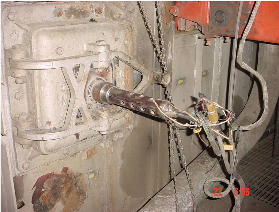
Figure 17. Corrosion probe inserted through the manhole at superheaters.
