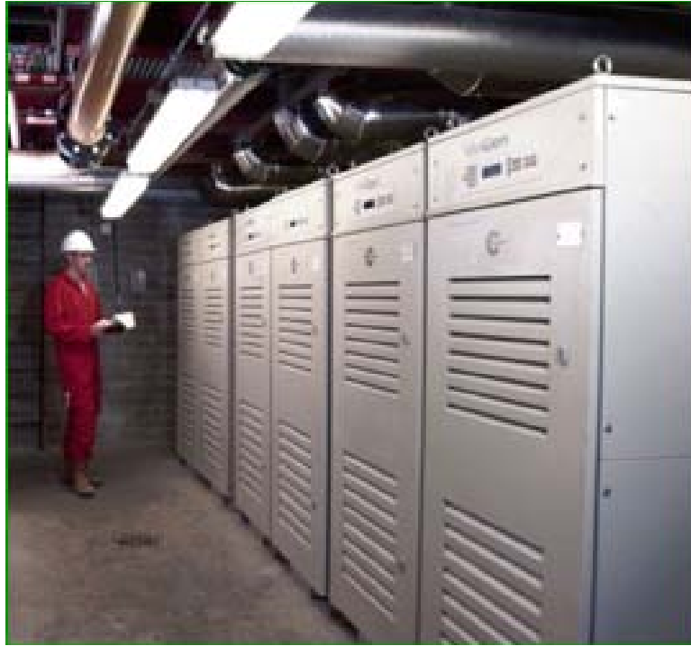
Figure 25. Six Capstone C60 Turbines at Guisborough Hall, UK
