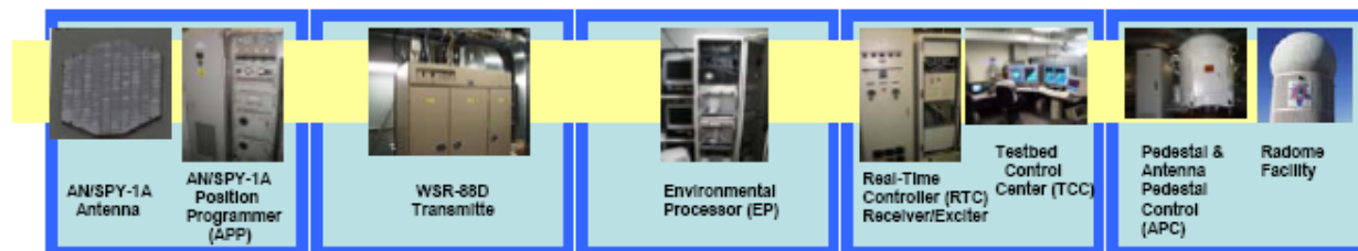
Figure 6. The National Weather Radar Testbed (NWRT) Equipment
