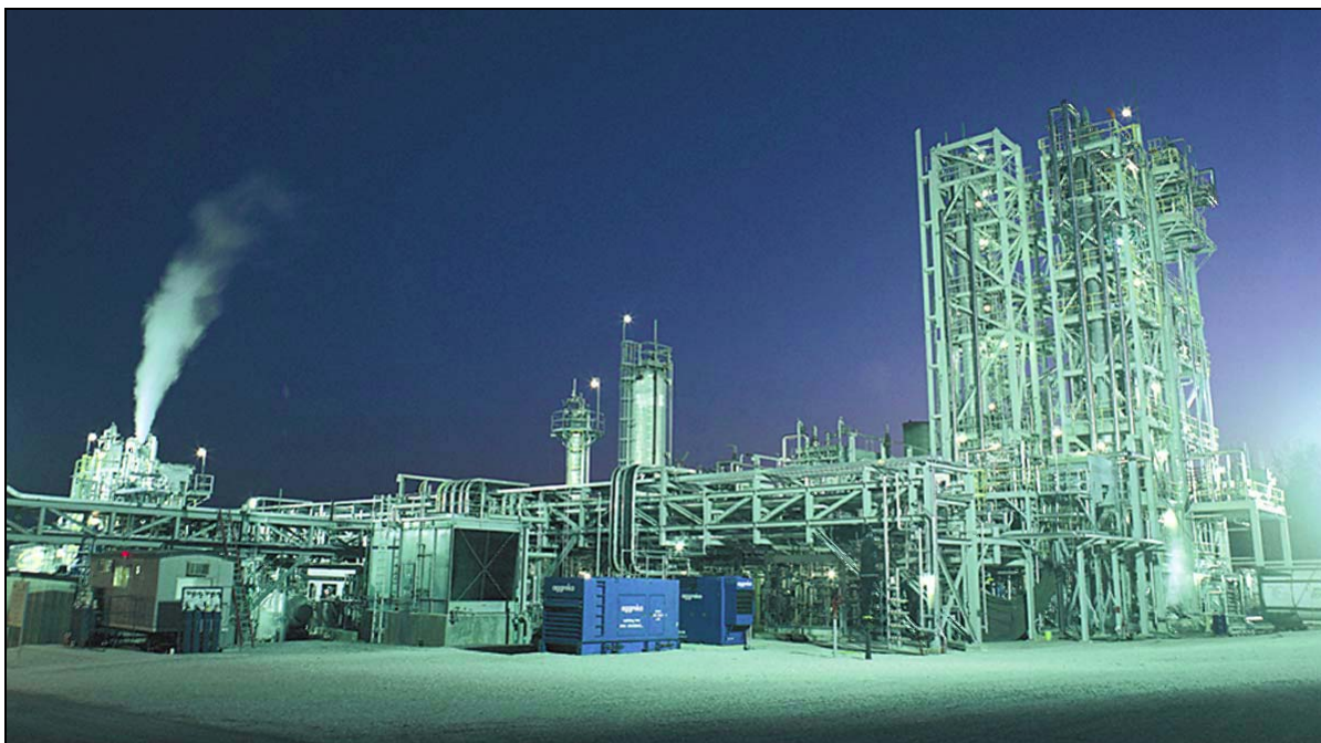
Figure 2: Syntroleum Pilot Plant in Tulsa Oklahoma [11]
