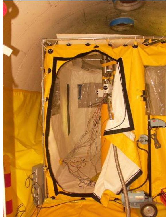
Figure 2.5.7. Secondary Containment Tent
