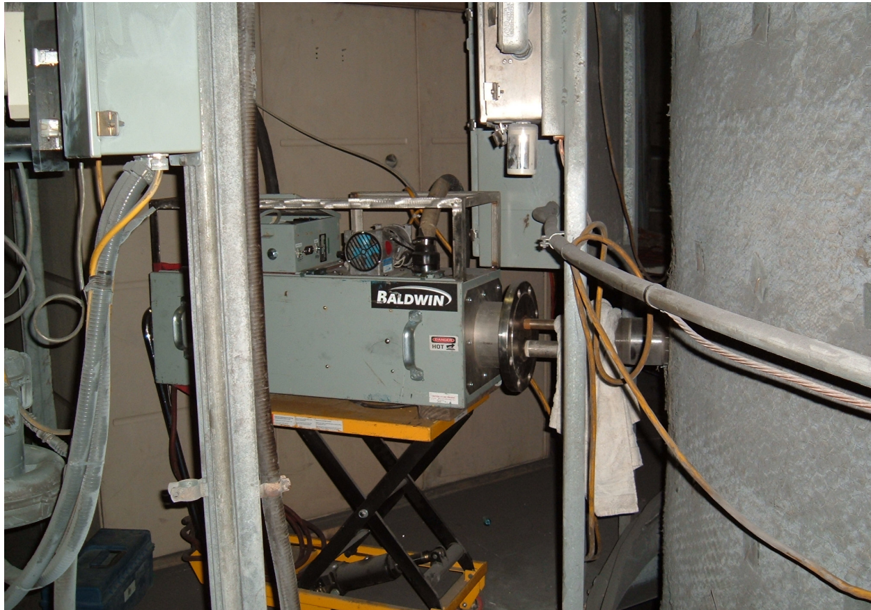
Figure 5.1-1 Inertial Separation Probe at Air Preheater inlet CMM Location
