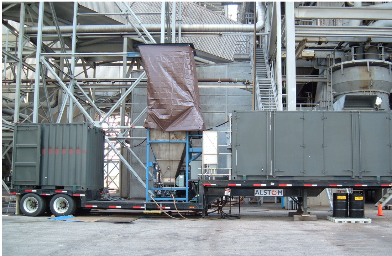
Figure 4.2-4 Mobile Mer-Cure™ Trailer Installed at Fayette Unit #3
