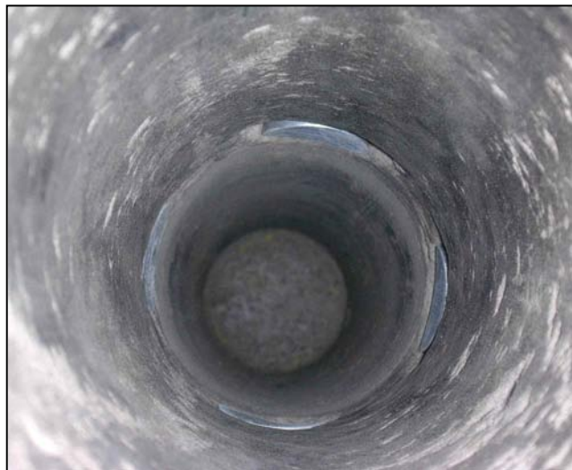
Figure 7. A view down the borehole in which the protective mounting pod for an embedded accelerometer may be seen at the top, flush with the wall of the borehole.
