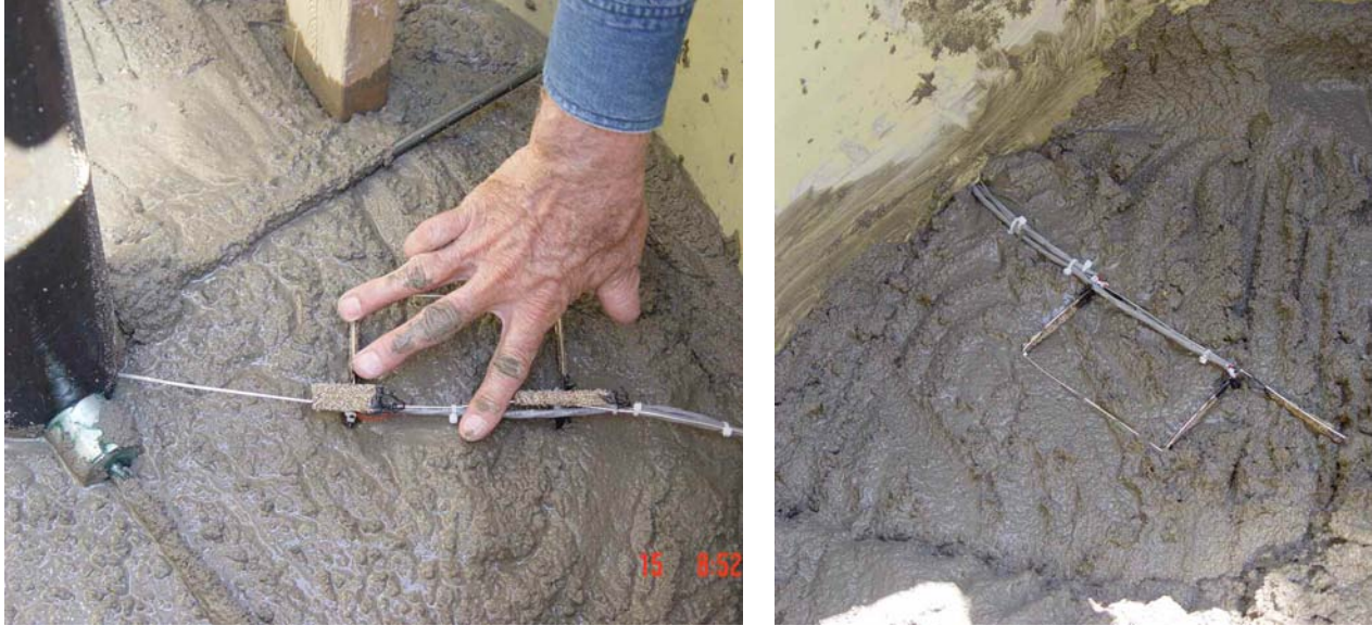
a b Figure 4. (a) Emplacing a set of strain gages at the mid-height of the pour (b) Gages in place showing the function of the emplacement jig for holding the correct distances and orientations.
