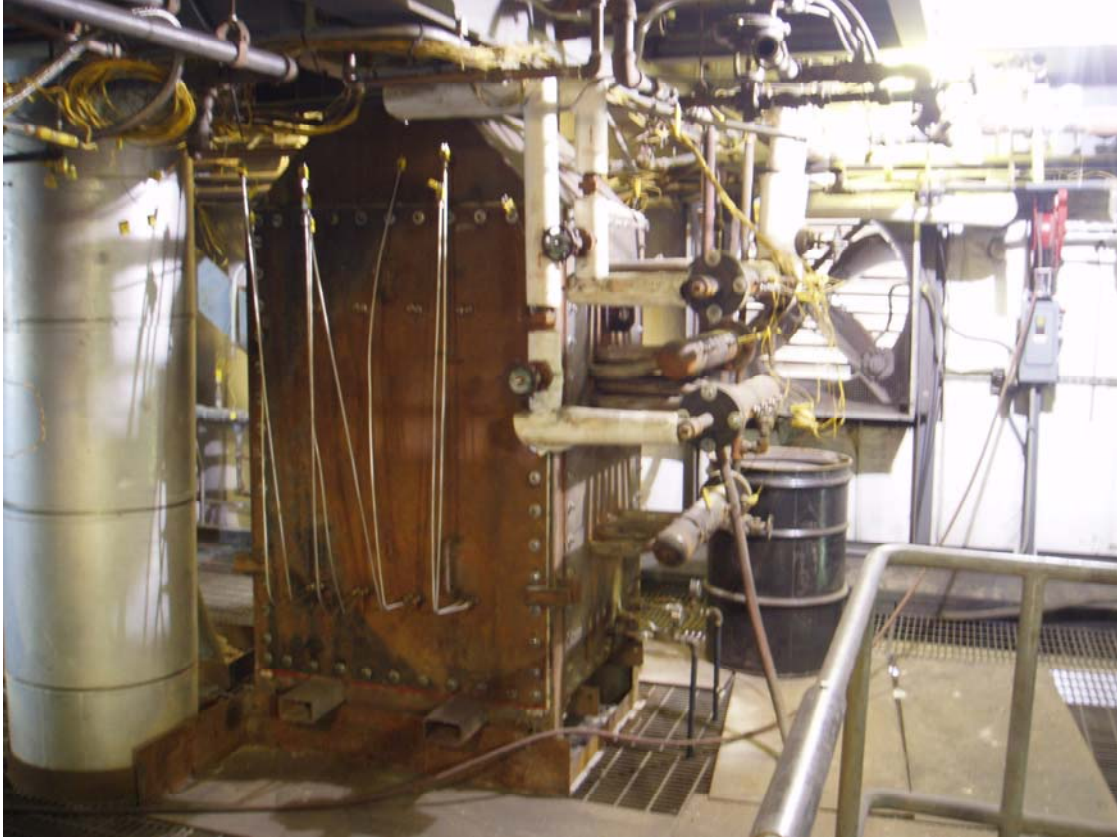
Figure 3.40: Moving Bed Heat Exchanger
