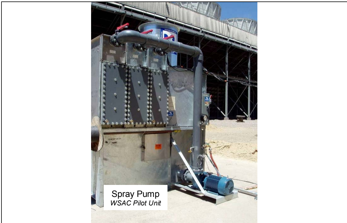
Figure 10-7 Spray Pump at WSAC Pilot Unit
