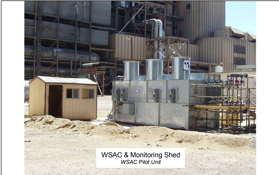
Figure 10-4 WSAC Pilot Unit and Monitoring Shed
