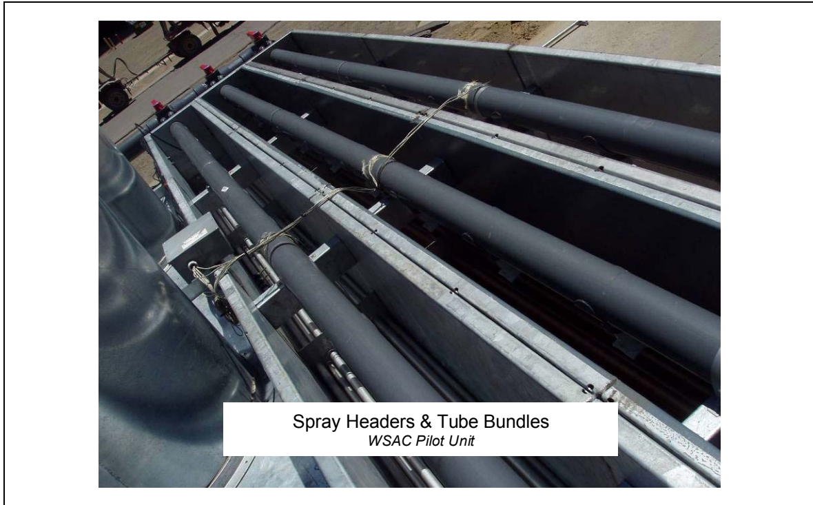
Figure 10-8 Spray Headers and Tube Bundles at WSAC Pilot Unit
