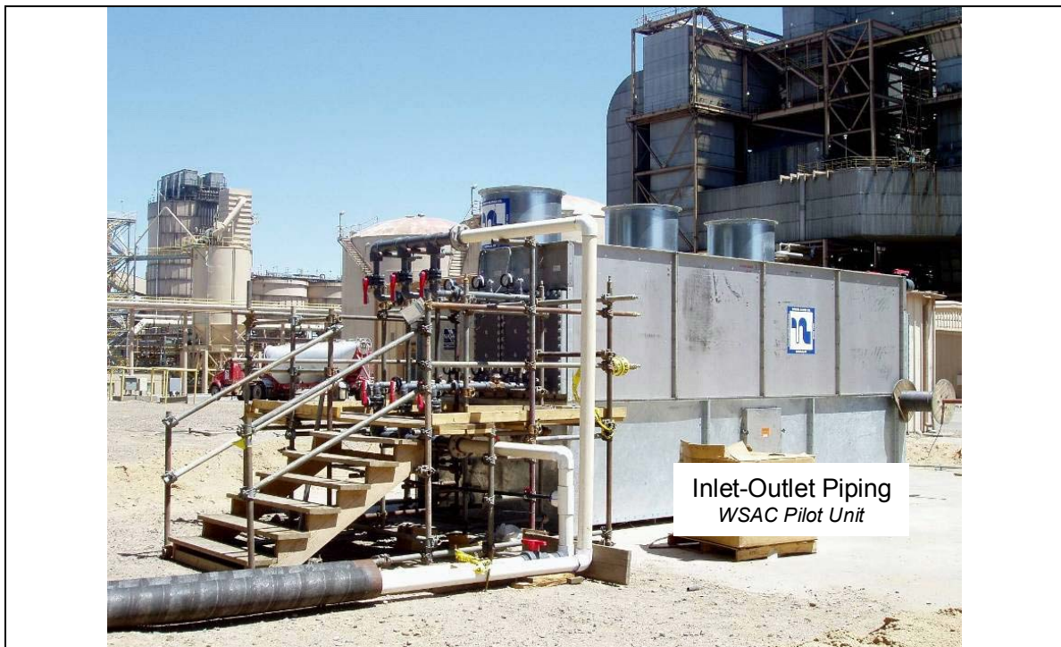
Figure 10-5 Inlet-Outlet Piping at WSAC Pilot Unit
