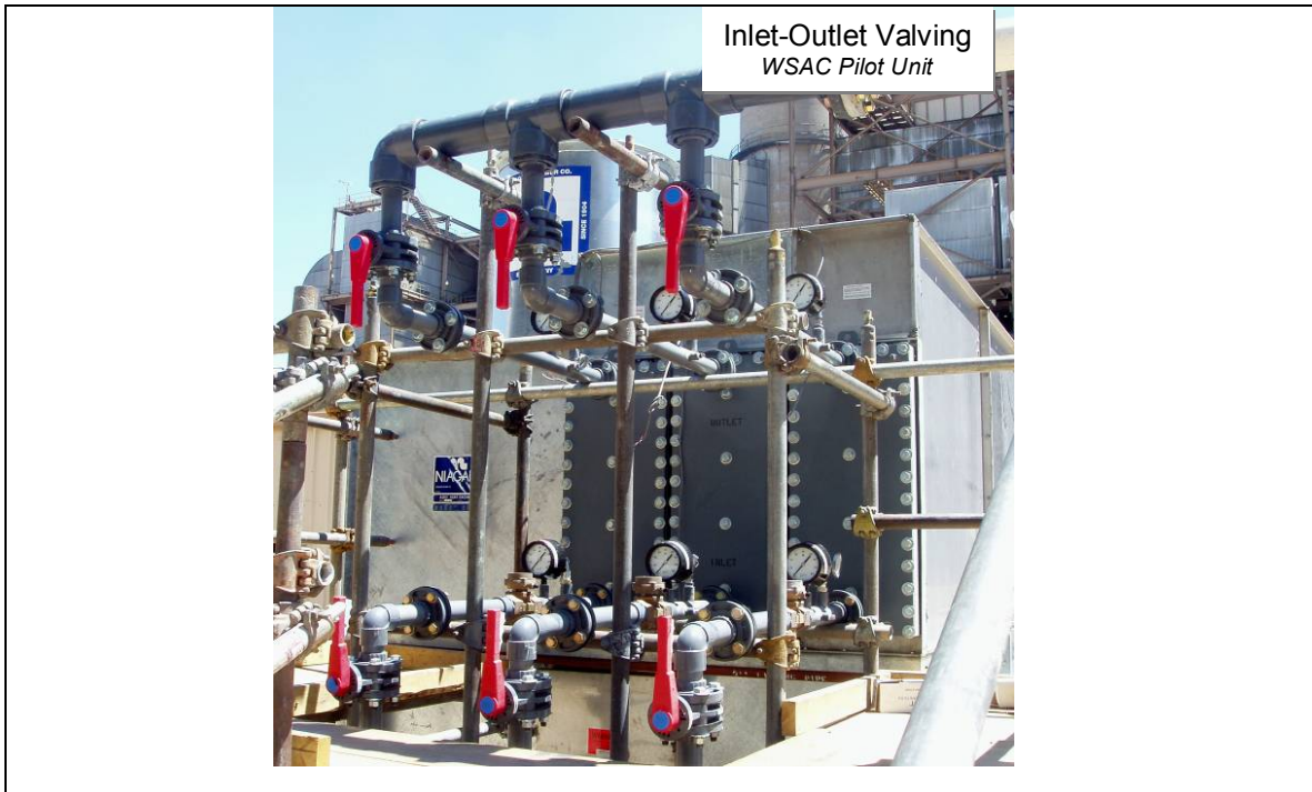
Figure 10-6 Inlet-Outlet Valving at WSAC Pilot Unit
