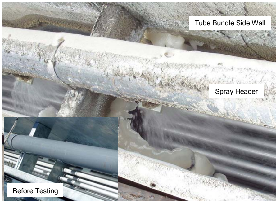
Figure 10-19 Mineral Scale Deposition - 316 SS Tube Bundle
