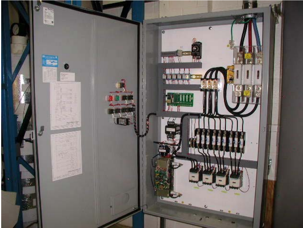
Figure 5.4 100kW power control panel
