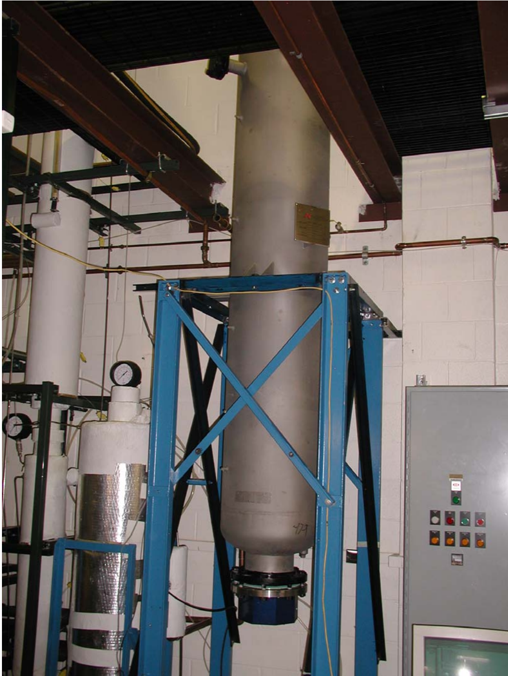
Figure 5.3 Steam generator tank installed. Inset: 100 kW immersion heater.
