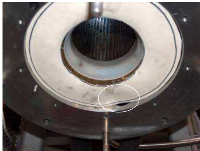
Figure 41: Drive end insulator plate. Oil flow area restricted.
