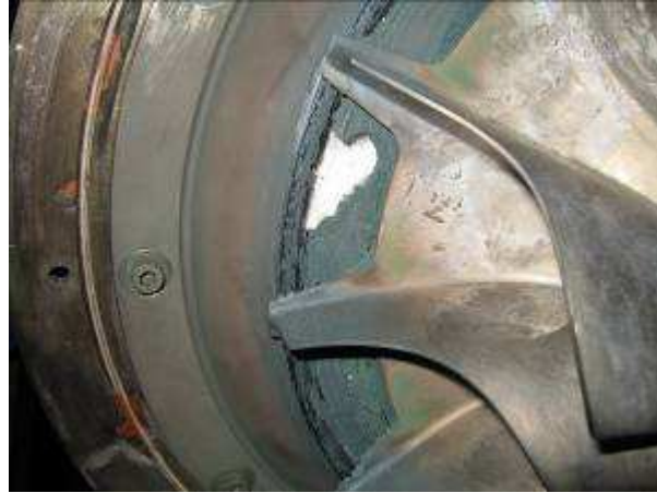
Figure 45: Turbine and Turbine Backplate Damage
