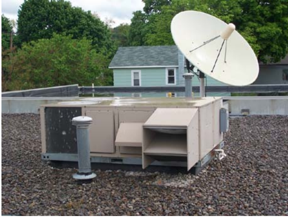
York Roof Top Unit on top of Willow
