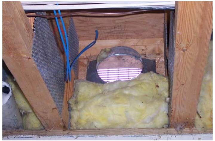
Abandoned Outdoor Air Intake
