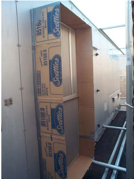
Figure A6-9. Munters Unit Ventilation Intake with Cardboard Duct to Direct Airflow
