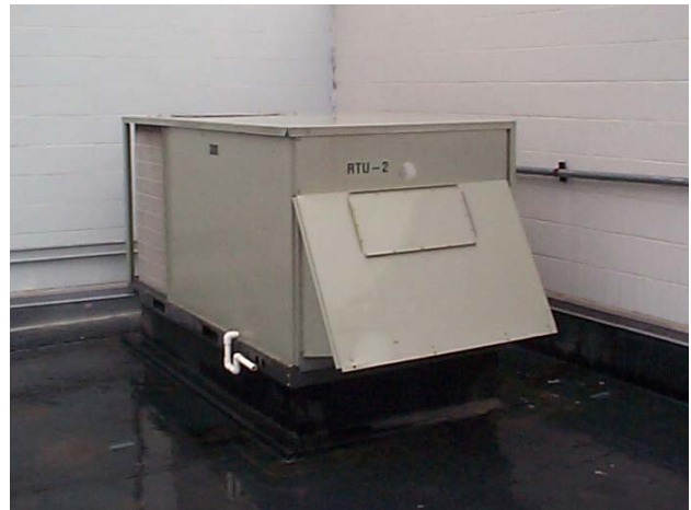
RTU-2 (Cooling Only – First Floor) Trane Model: TCD102C30AAB
