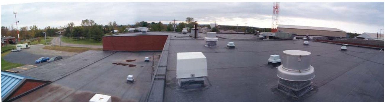
Figure A11-12. Sealed Exhaust Fans for Blower Door Test
