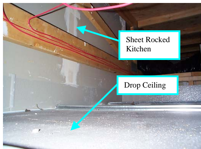
Sheet Rocked Wall in Kitchen Plenum
