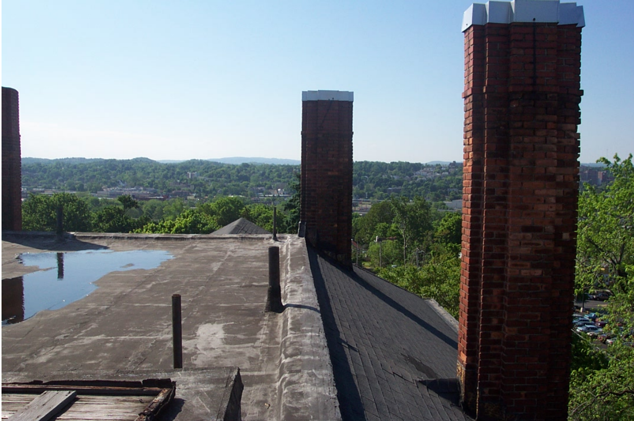
Figure A17-5. Corinthian Club Roof – Built Up Roof and Shingled Roof Transition
