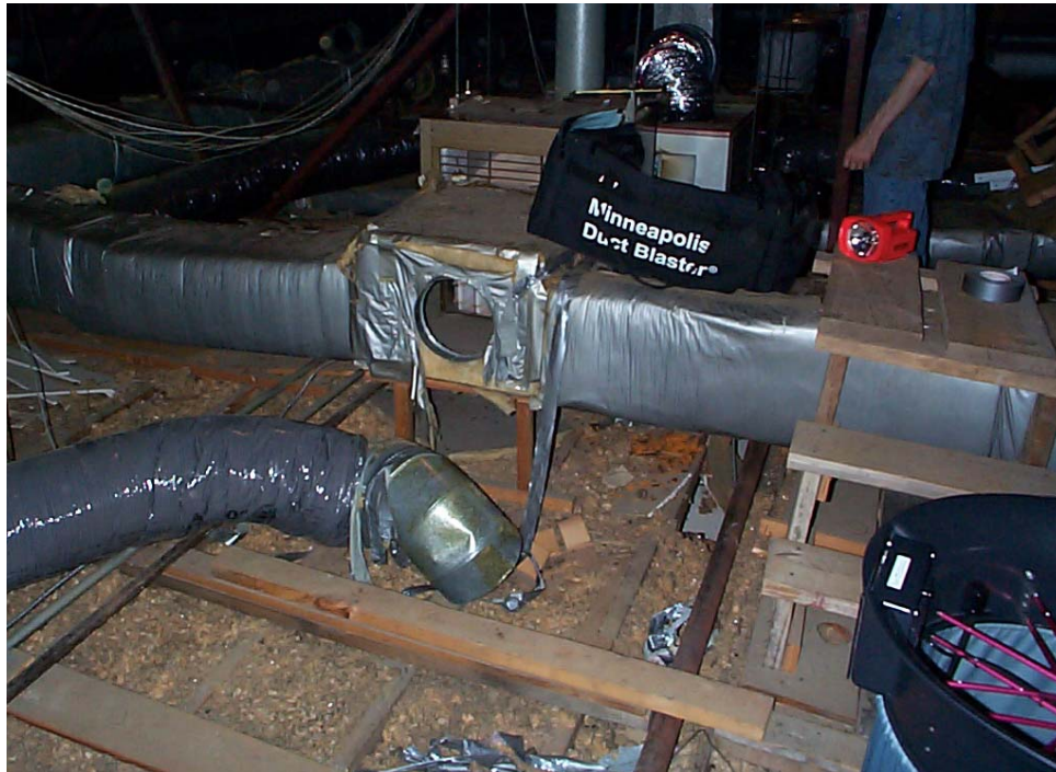
Figure A4-17. Photo Showing Disconnected Supply Duct on AHU #2 (Reconnected for Duct Testing)
