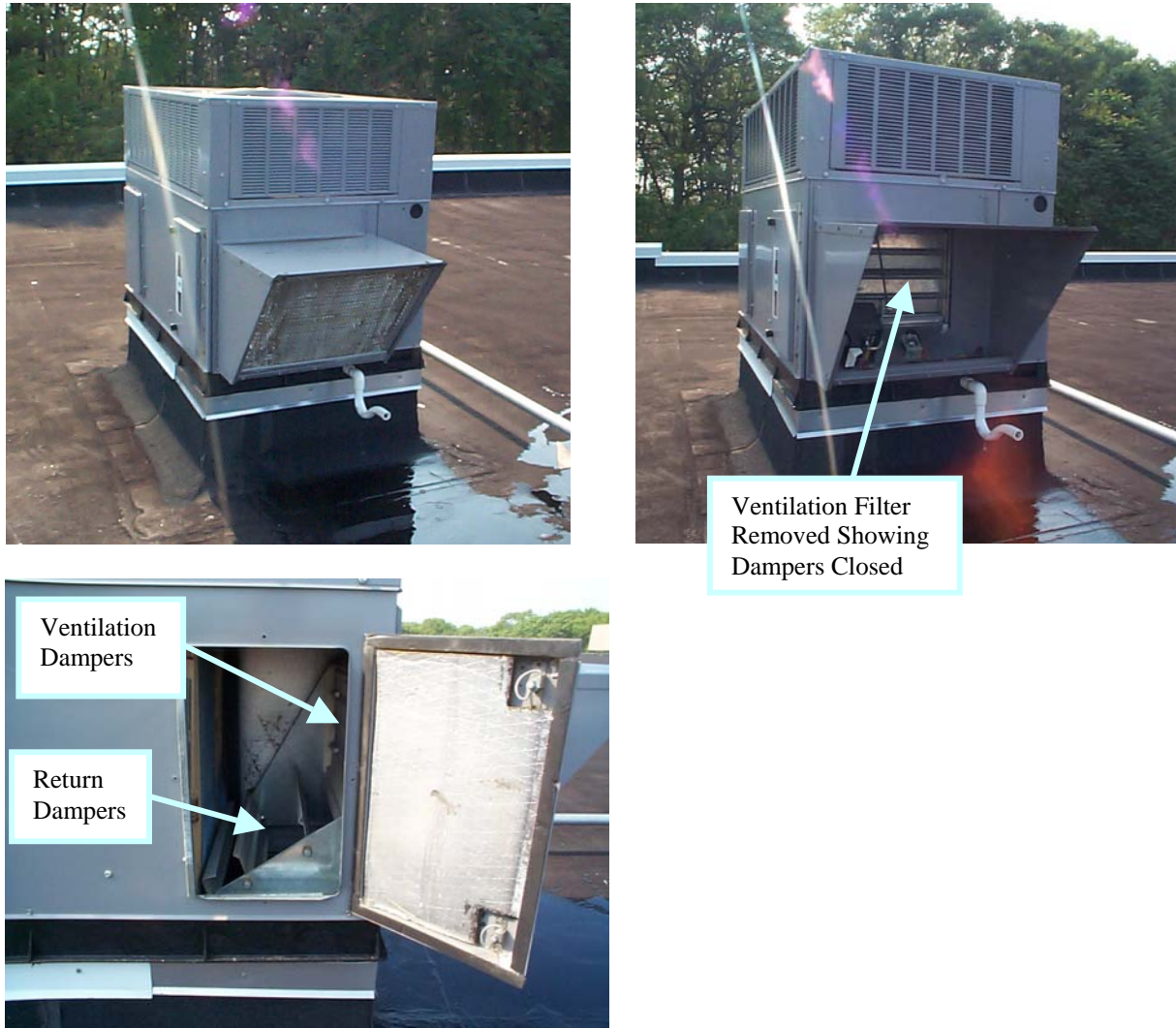
Figure A6-11. RTU-4 with Operating with Ventilation Dampers Closed
