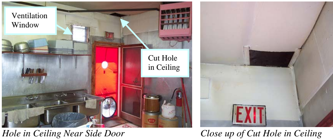
Figure A2-11. Source of Leakage (Ventilation Air) in Chinese Restaurant
