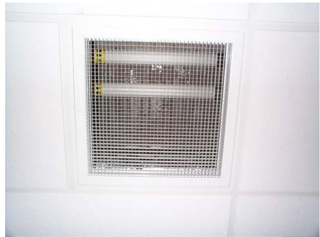
Typical Return Grill to Ceiling Plenum
