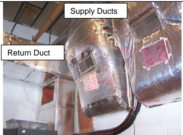
Supply Ducts and Cooling Coils
