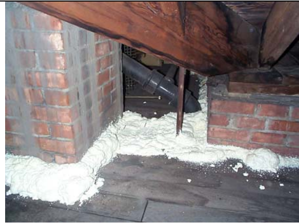
Large Area Leak Around Drain Plumbing
