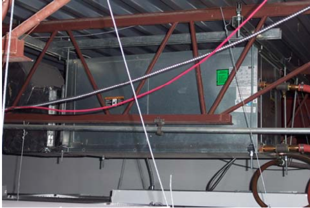
Figure A12-5. One of the WSHPs Serving Office Section
