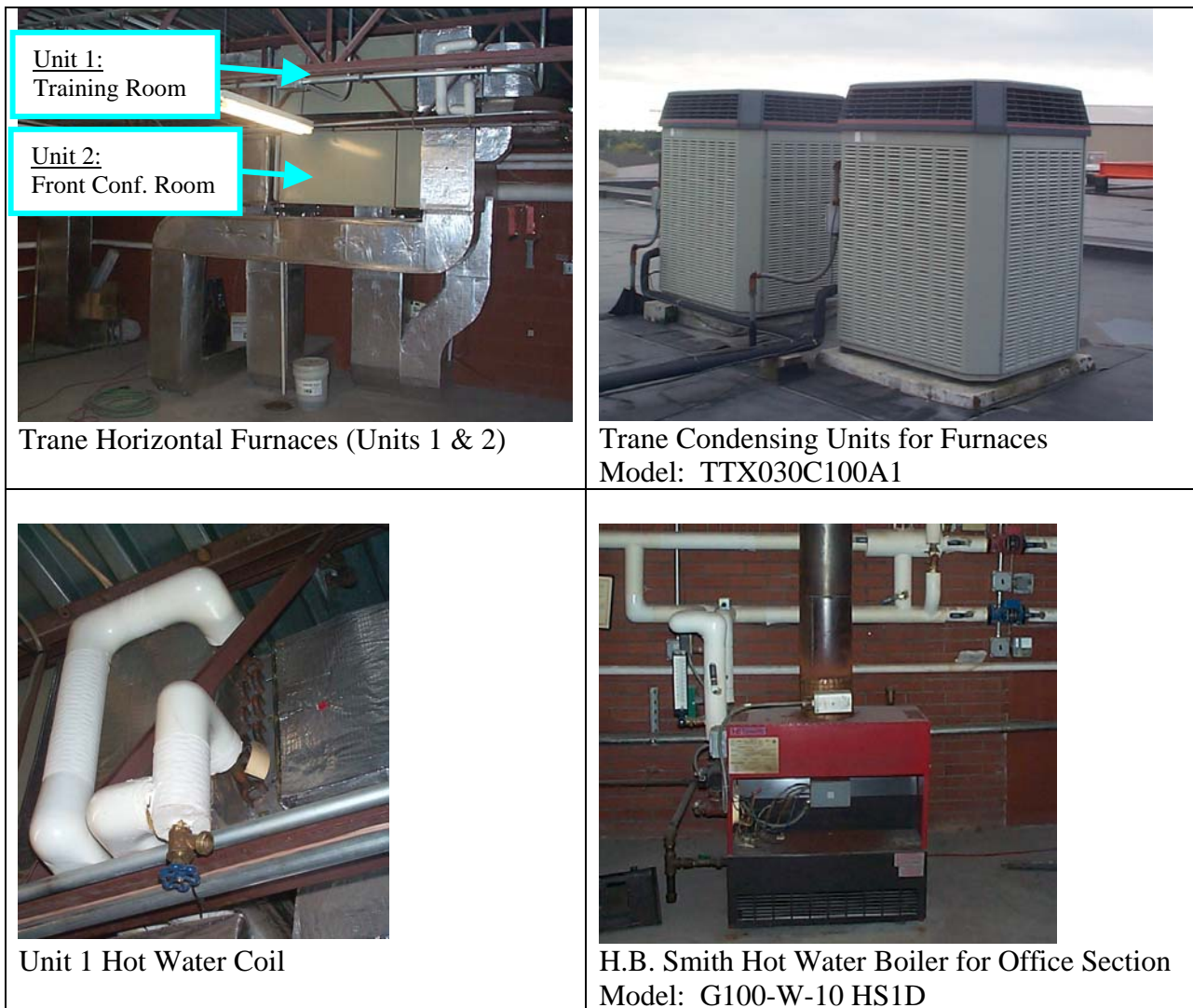
Figure A11-6. HVAC Equipment for Office Section of Building
