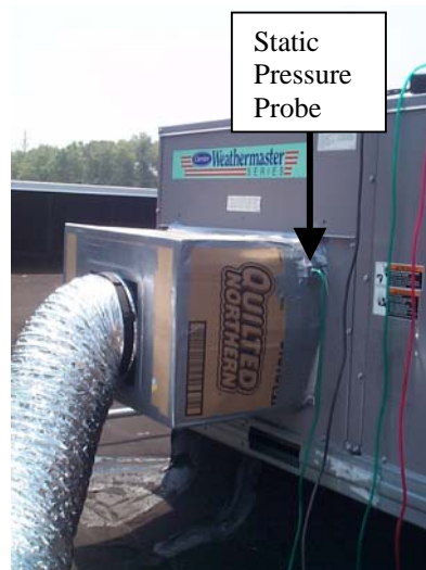
Static Pressure Probe in Same Location With Duct Blaster Connected
