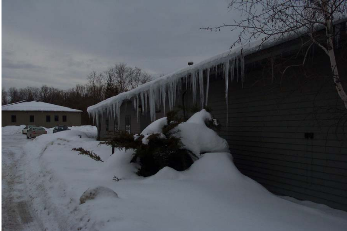
Figure A2-32. Ice Dams Formed from Leakage to the Attic
