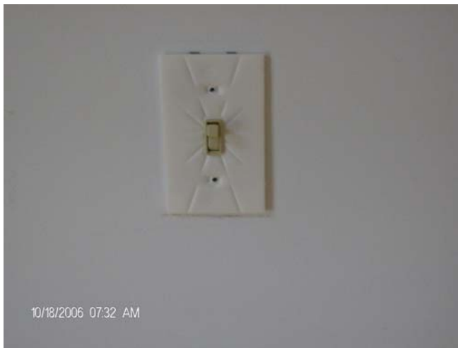
Electrical Switch Outlet (Ceiling Lights)
