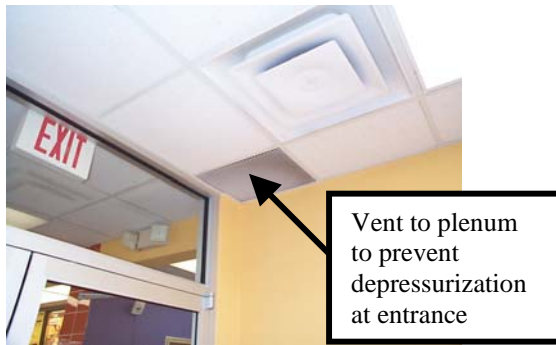
Figure A9-13. Vent to Plenum at Entrance
