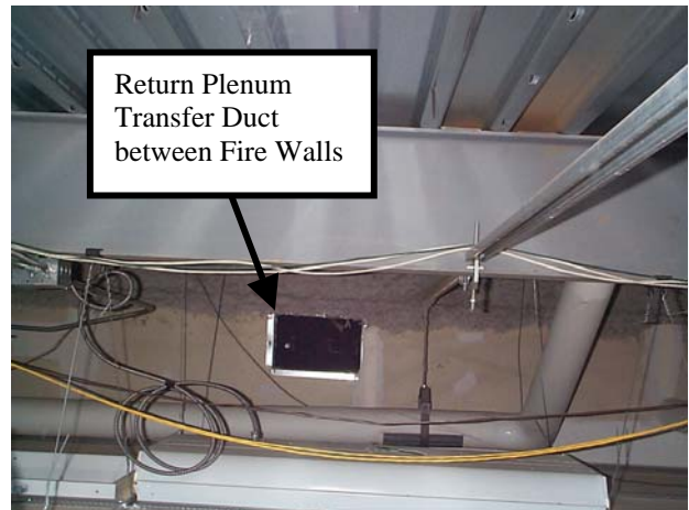
Plenum Transfer Duct Between Interior Walls
