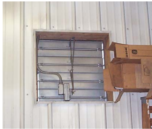
Exhaust Damper (West Wall)
