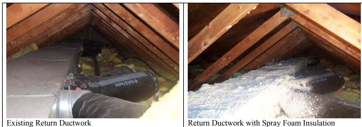
Figure 3-6. Return Ductwork in Attic Space
