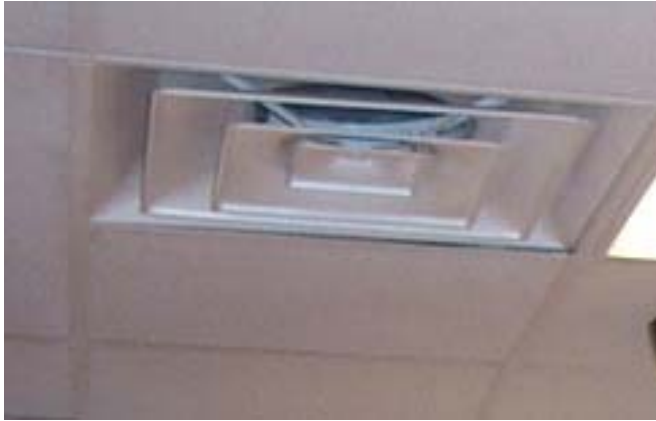
Figure A7-9. Four Cone Diffuser in Drop Ceiling
