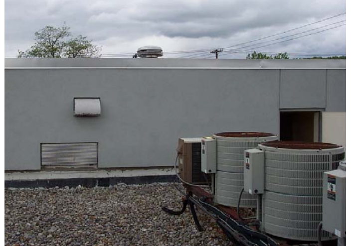
Carrier Condensing Units Serving AHUs on top of Willow (3 operating, 2 abandoned)
