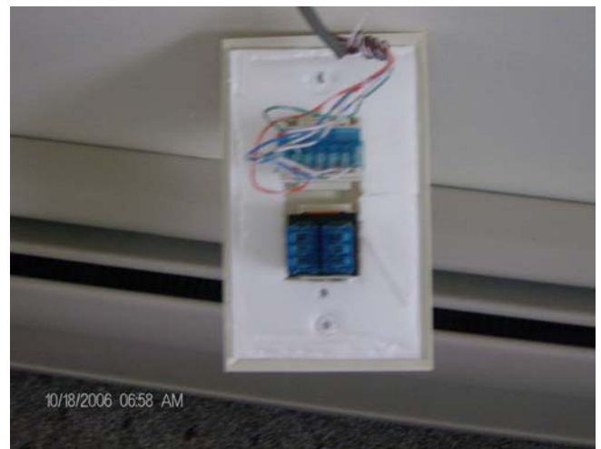
Communications Outlet (Phone and Internet)
