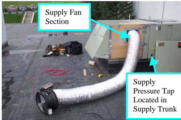
Duct Blaster Connected to RTU-1
