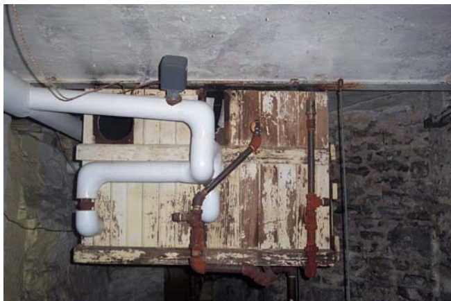
Figure A17-9. Steam Coil without Fan (natural convection induces airflow from the basement)
