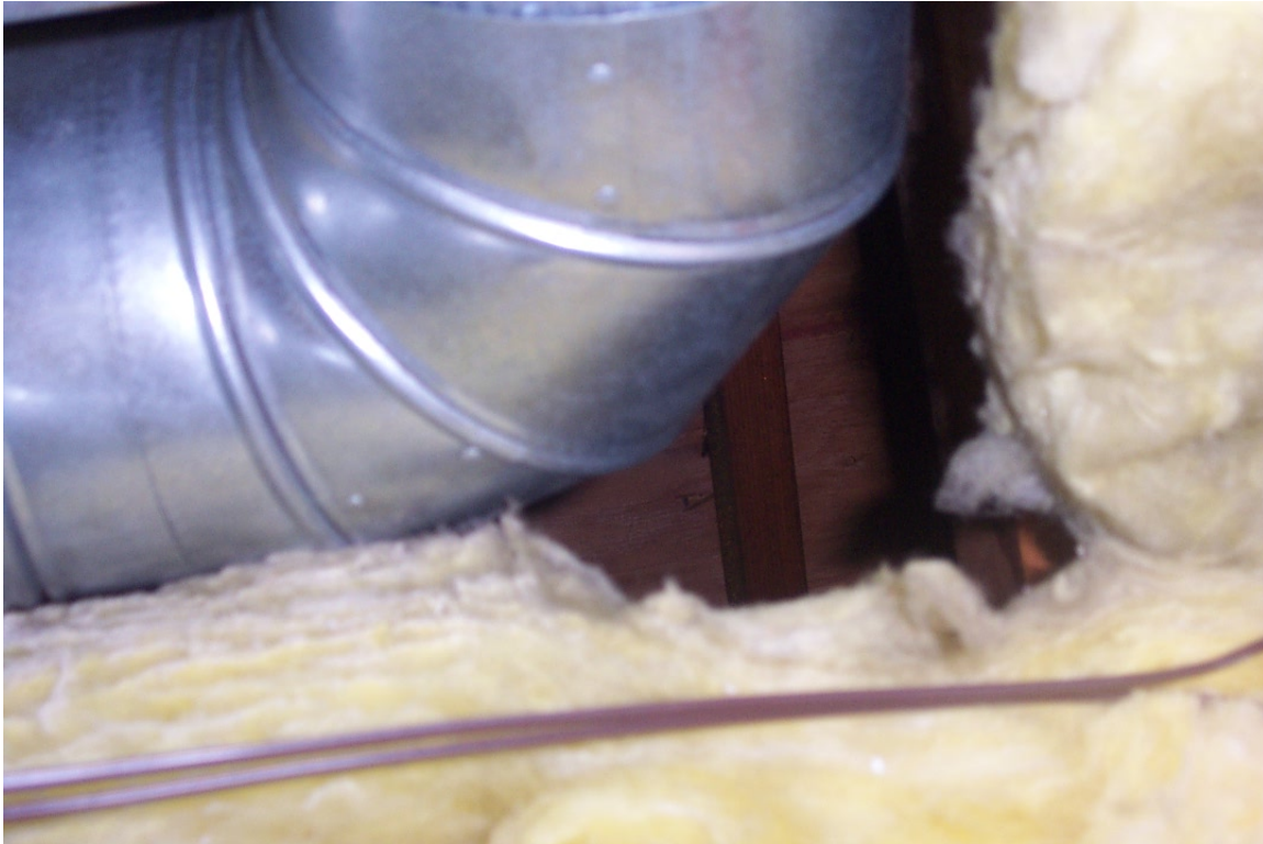
Figure A2-31. Hole in Fiberglass Insulation (Thermal and Air Barrier) – Viewed from Below
