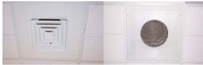
Typical Supply and Return Grill
