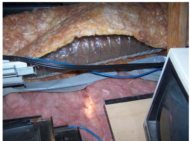
Insulation coming off of the flex duct
