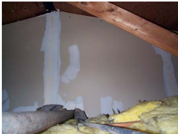
Figure A2-7. Firewall in Attic Between the Restaurant (Site 3) and Office (Site 2) Sections
