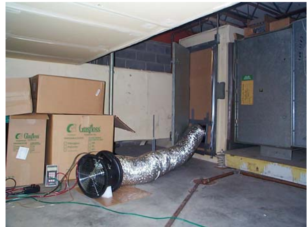
Duct blaster connected to VAV System for depressurization
