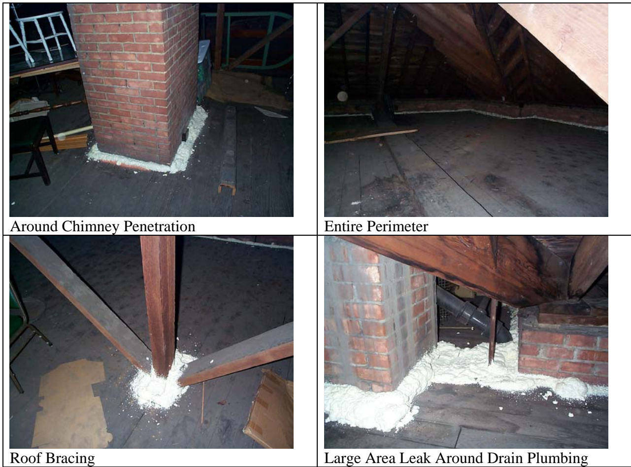
Figure A17-32. Different Types of Leaks Sealed with Expandable Foam
