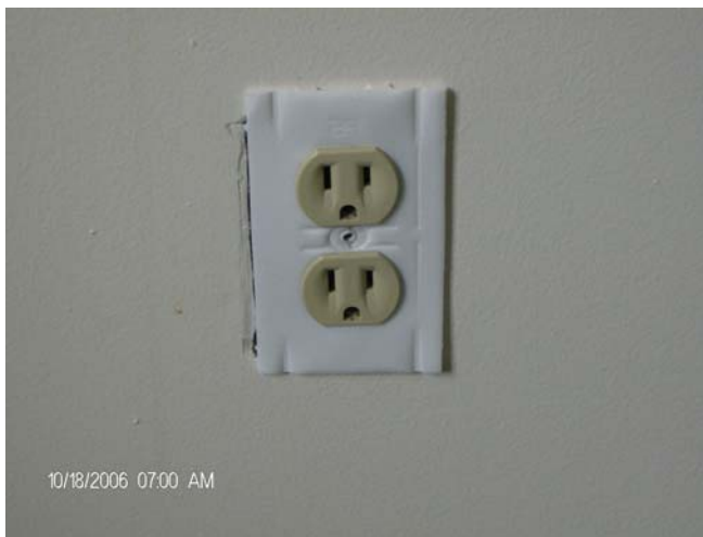
Electrical Power Outlet
