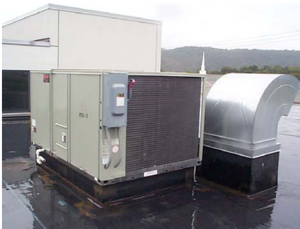
RTU-3 (Cooling Only – First Floor) Trane Model: TCD150C30ACA
