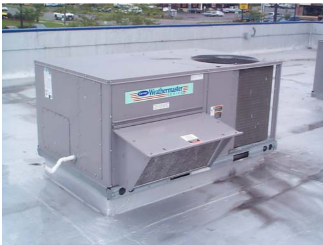
Typical Rooftop Unit
