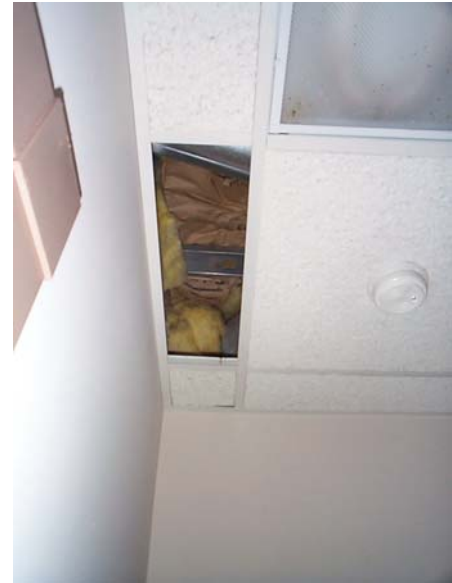
Missing Ceiling Tile Near Closet
