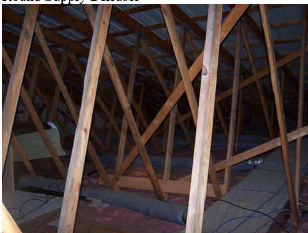
Ductwork above insulated Ceiling Framework
