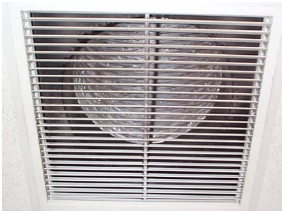
Return Grate with 18-inch Return Duct
