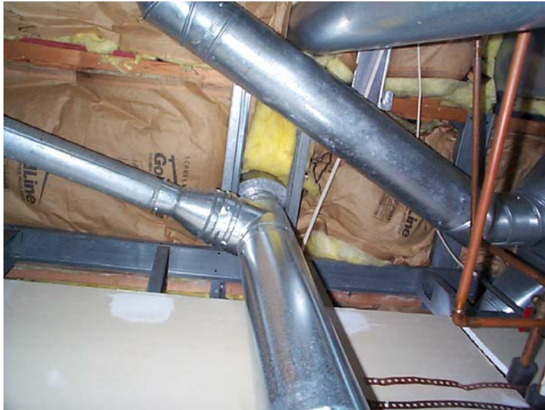
No Ceiling in Closet Enclosing AHU and Water Heater
