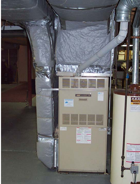
Lennox Furnace and A-Coil Unit
