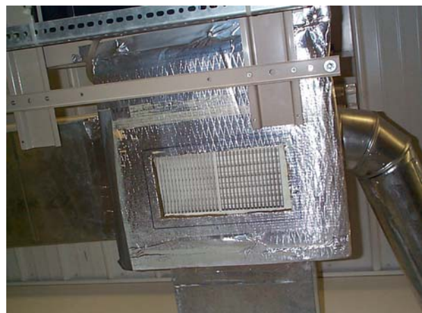
Supply Grill on Underside of Furnace
