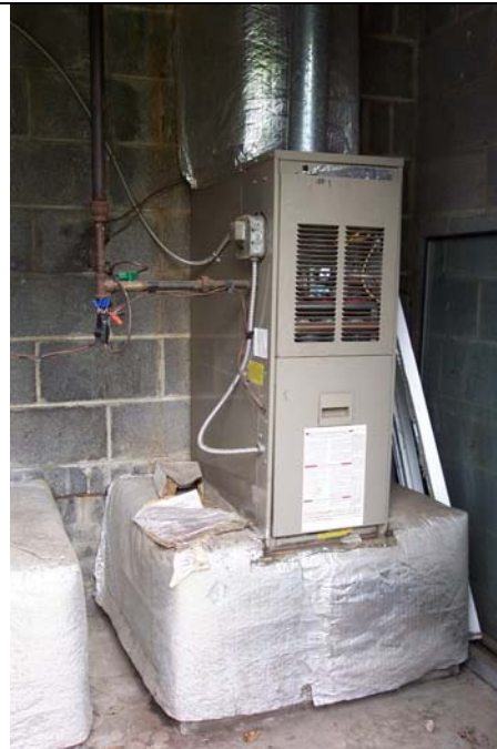
Furnace on top of Return Air Plenum in Shed
