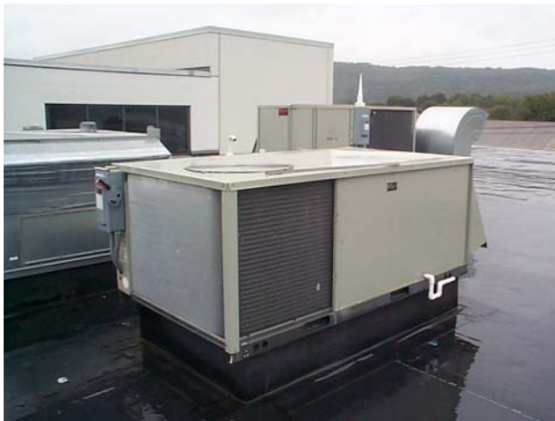
RTU-1 (Cooling Only – First Floor) Trane Model: TCD090D30ABC
