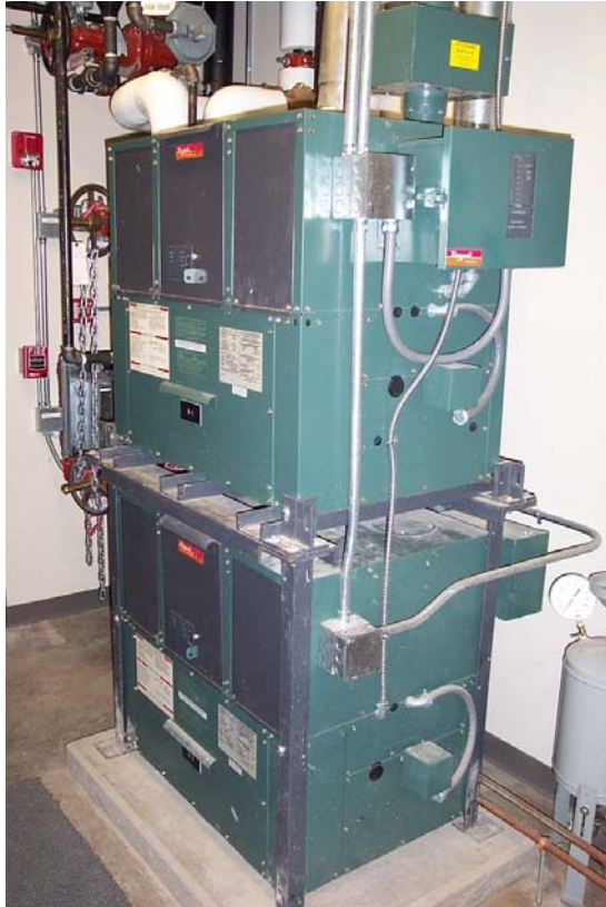
Boilers (B-1 & B-2) Raypak Model: H3-0302
