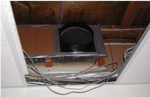
Duct Blaster fitting on Return Duct in Plenum
