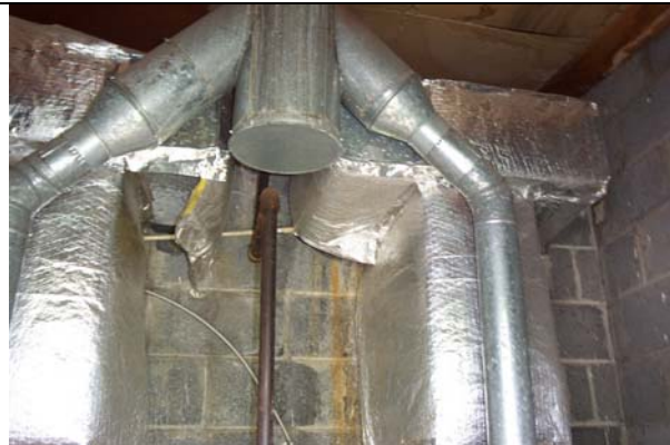
Furnace Flue Vents and Supply Air Ducts
