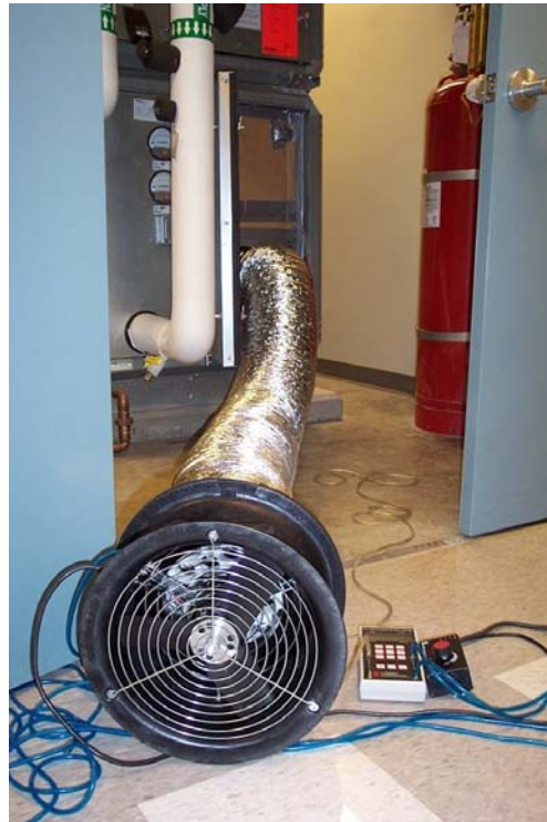
Duct Blaster Connected to Supply Section
