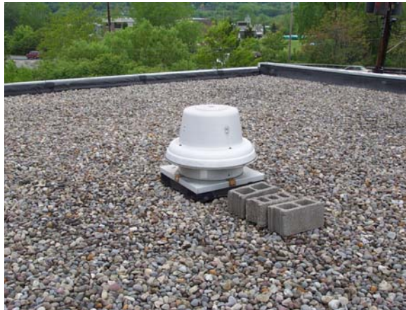
Exhaust fan “submerged” in New Roof & Insulation – Willows Second-story roof
