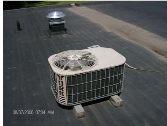
York 3.0 ton Condensing Unit (AC5)
