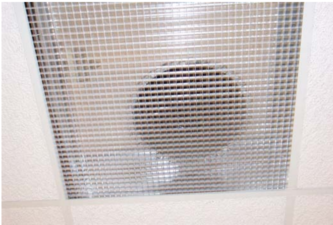
Return Grate with Single 12-inch Return Duct
