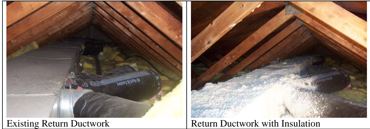
Figure A2-34. Return Ductwork in Attic Space
