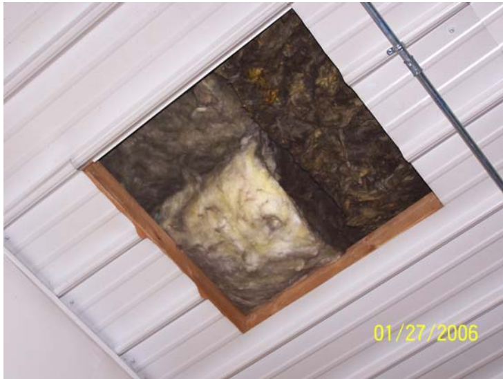
Figure A22-5. Uncovered Opening in Metal Ceiling in the Repair Shop
