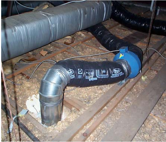
Figure A4-9. One of Two Thermostat Controlled Inline Duct Fans
