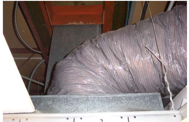
Flex Duct Takeoff to Damper Vent through Roof
