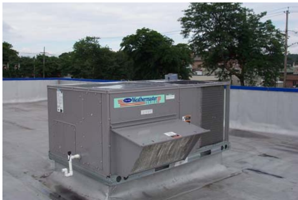
Typical Rooftop Unit
