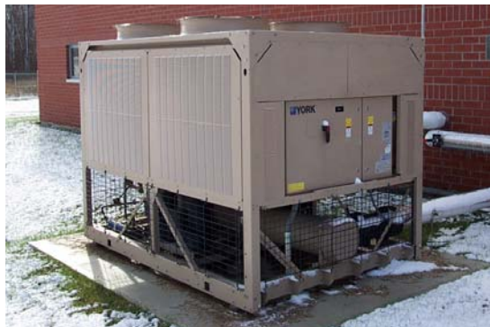
Chiller (CH-1) York Model/PIN: YCAL0050EC46XCASDTXLTXBLXXXX45SX1XXXXDXSAXXXXX3BXXLXNHXXXXXX
