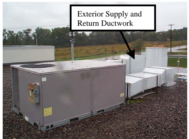
RTU-4 (Cooling and Hot Water Coil for Heating – Second Floor) Carrier Model: 50TJ-009-501
