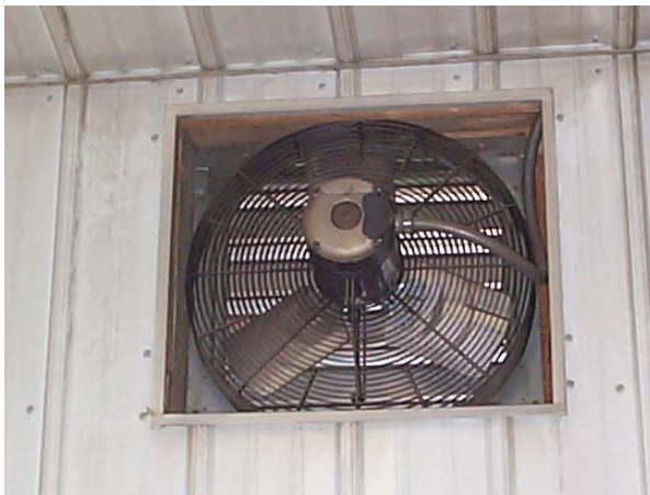
Exhaust Fan (South Wall)
