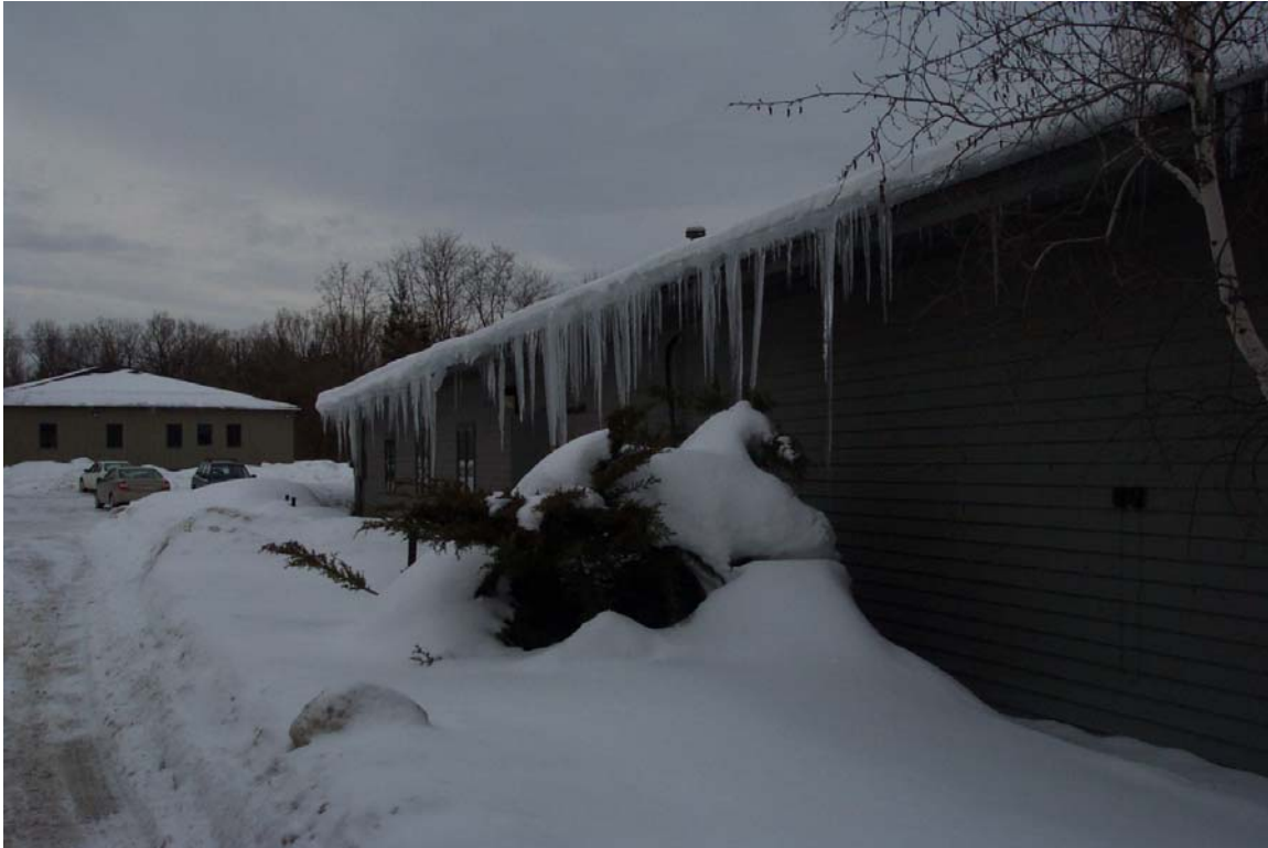
Figure 3-4. Ice Dams Formed from Leakage to the Attic
