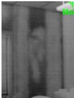
Inside View Wall Void In Eastern Office
