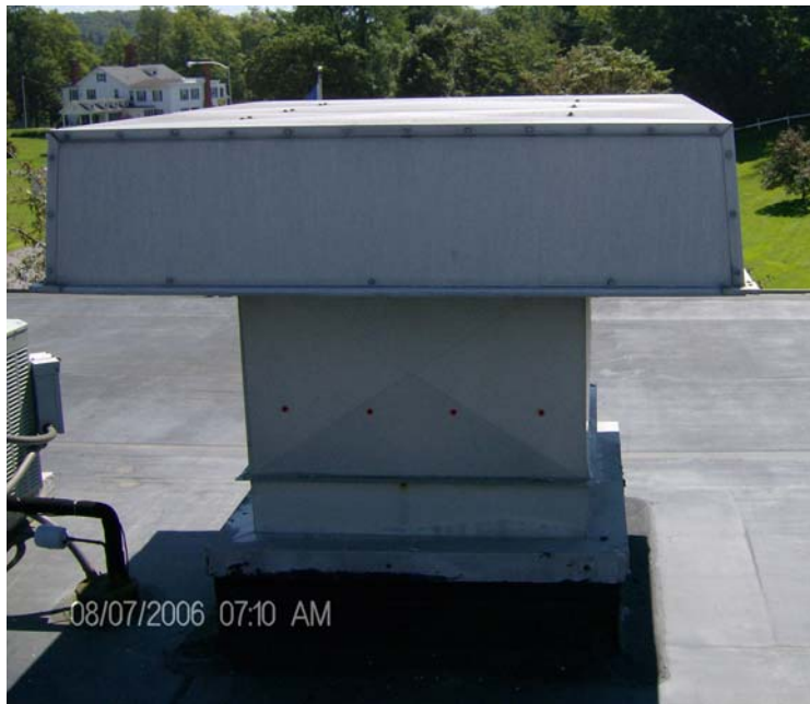
Figure A24-8. Makeup Air Intake Showing Traverse Points
