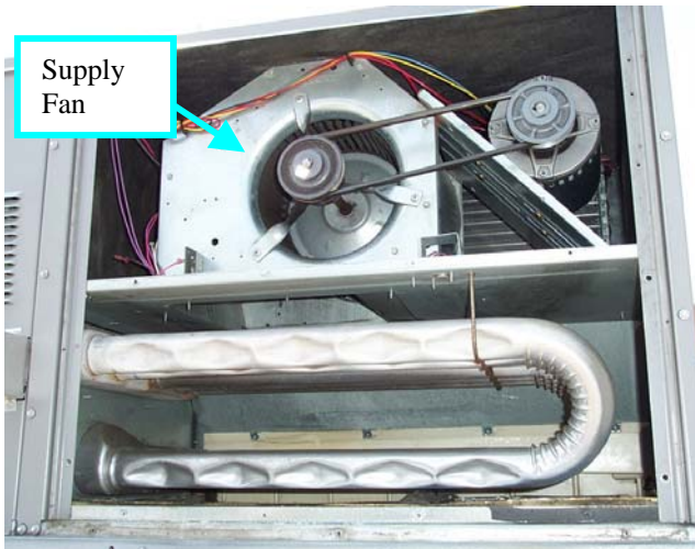
Unblocked Supply Side
