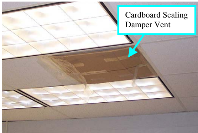
Barometric Damper Sealed Off
