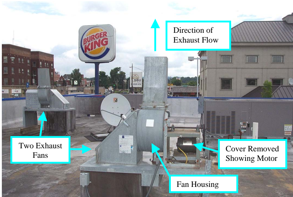
Figure A7-11. Grill and Fryer Exhaust Fans
