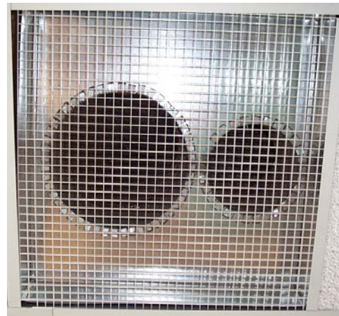
Return with 8 and 12-inch Return Ducts
