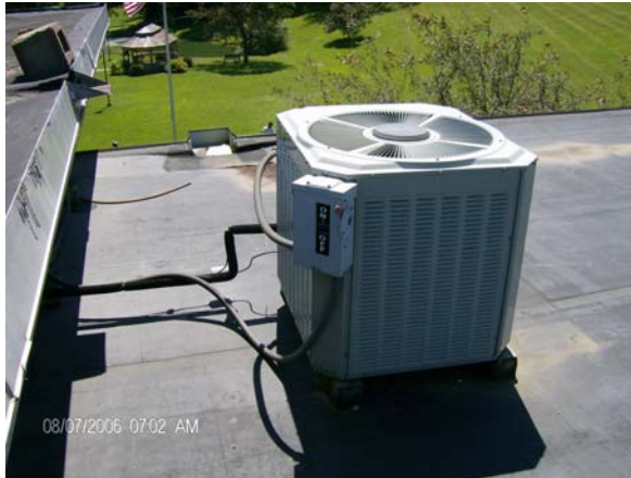
Trane 1.5 ton Condensing Unit (AC1)
