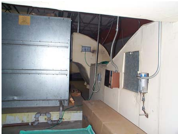
Variable Air Volume System
