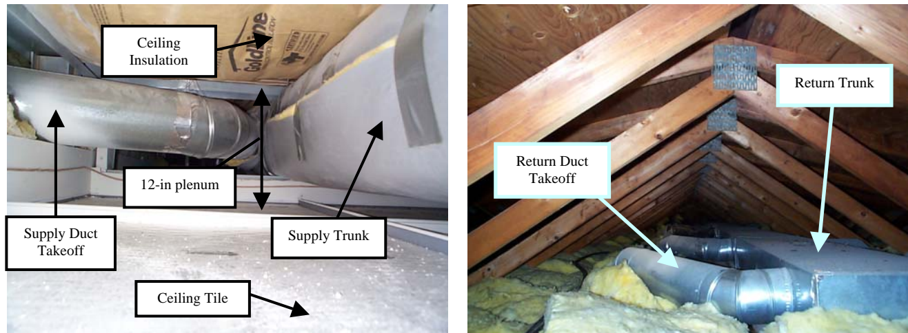
Figure A2-6. Office Section: Ceiling Plenum with Supply Ductwork and Attic with Return Ductwork
