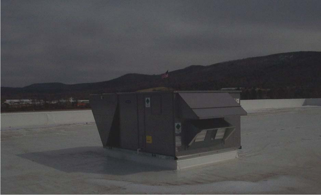
Figure A23-5. RTU Located on Roof / Dropdown Diffuser for an RTU Inside Store
