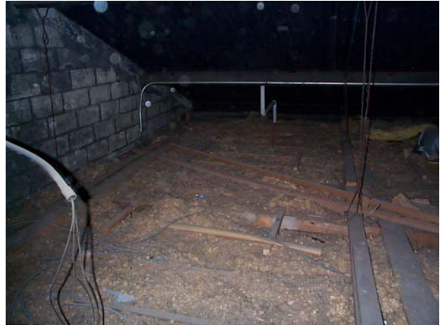
Rock Wool Ceiling Insulation
