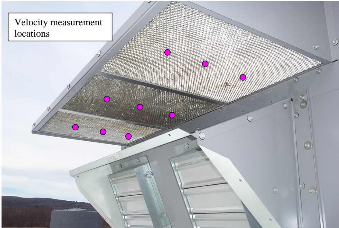
Figure A23-8. Fresh Air Intake Hood on each RTU
