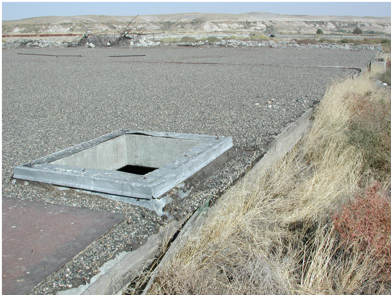
Figure 5. 183-F East Clearwell Open Hatch.
