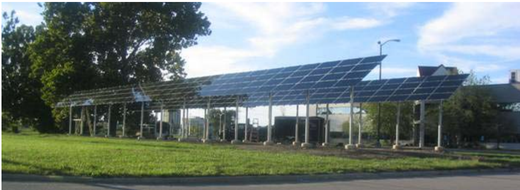
Figure 1.8: Two 6kW pole mounted solar arrays.
