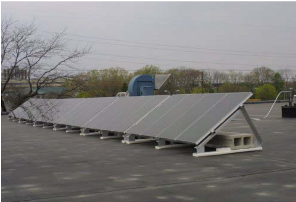
Figure 1.7: 1kW roof mounted solar array.
