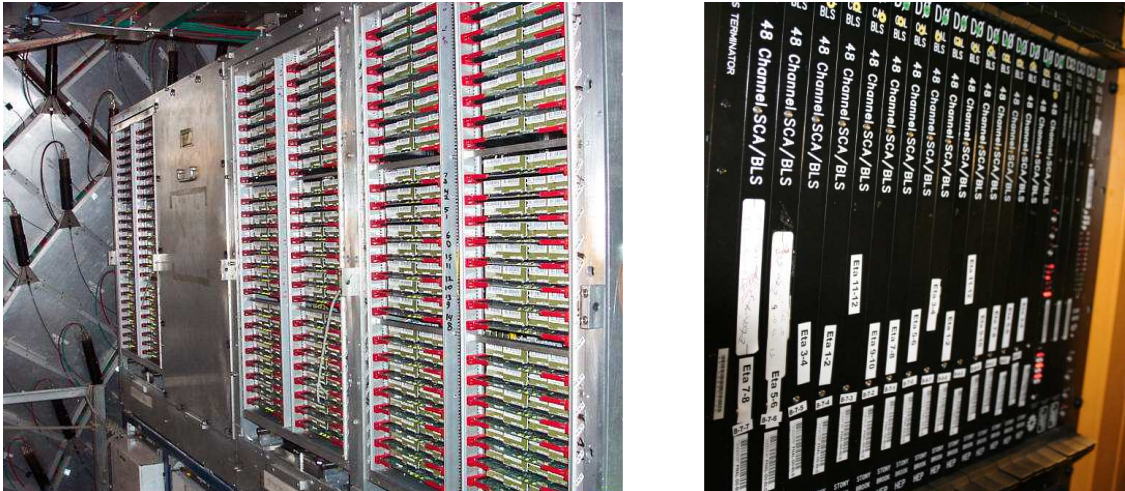
Figure 3.19: Pictures of the calorimeter preamplifiers on top of the endcap calorimeter vessel [62] (left) and BLS boards located on the DØ platform beneath the calorimeter [70] (right).
