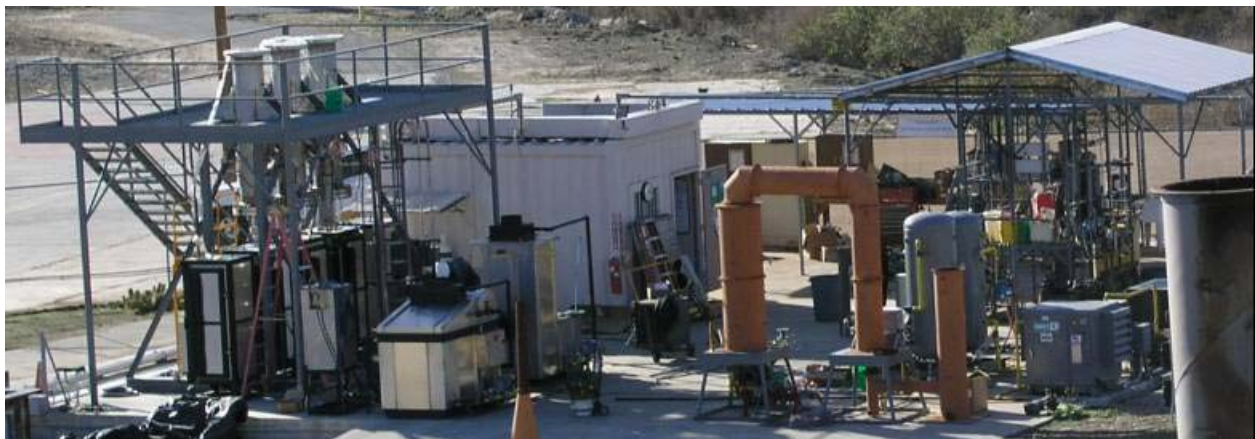
Figure 2-15. Photo of assembled pilot plant system.
