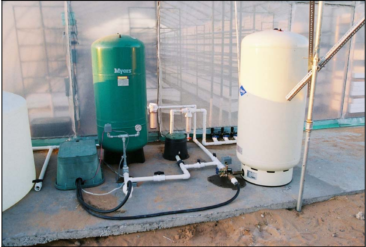
Figure 3-5 Water system on south end of greenhouse facility. Edge of white 550-gallon storage tank is at far left. Pressure tank in middle supplies irrigation system. Pressure tank on right supplies a faucet on the north end of the facility for seed preparation, tray cleaning, and general use. Rectangular utility box houses the pumps. Round utility box houses the irrigation system flow meter.
