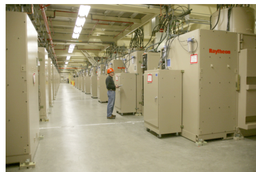
Figure 1. Completed Capacitor Bay with 48 modules, capable of storing ~100 MJ of electrical energy for flashlamps.
