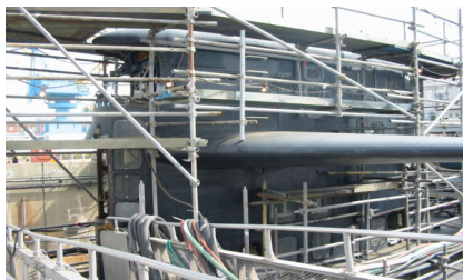
Sail of Ex-Portsmouth 688 Class Submarine with Black Epoxy Coating on Exterior Surface
