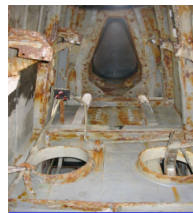
Internal Aft Sail Corrosion
