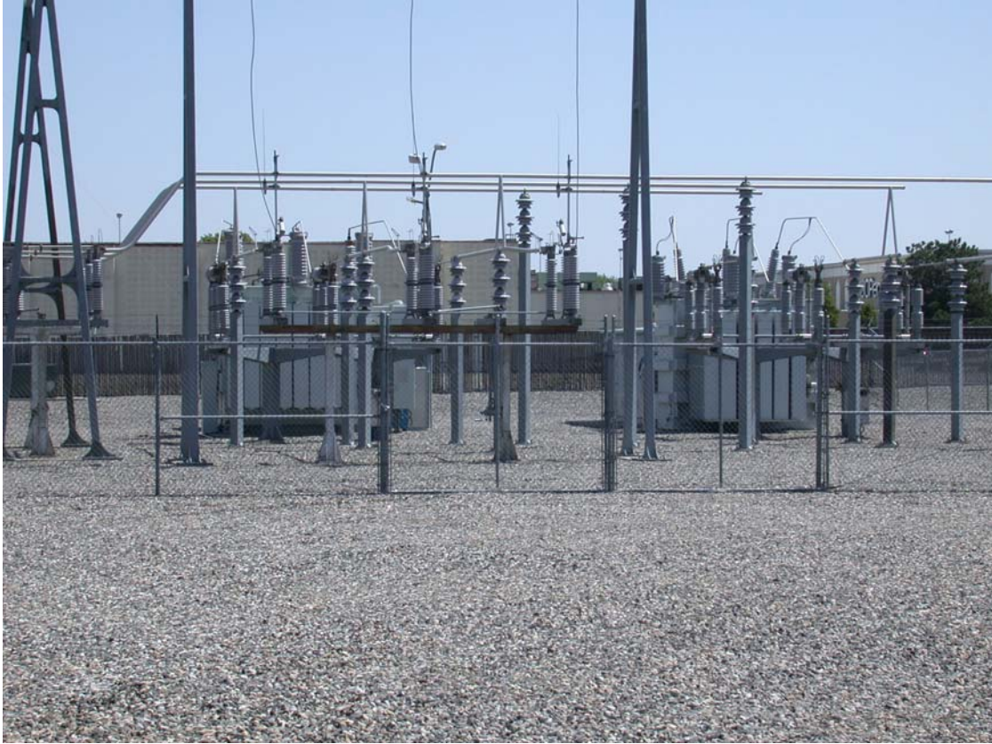
Figure 4.2. Picture of Vista substation
