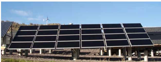
Fig. 1. Typical OTF rack mounted PV system.
