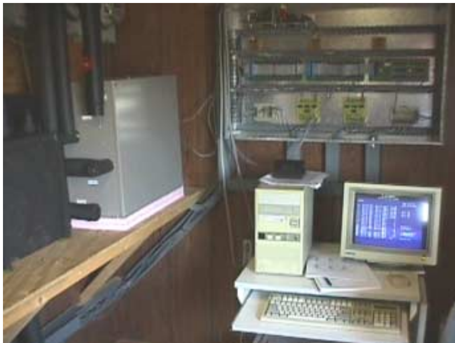
Figure 3. Interior of data acquisition shelter — grout performance comparison.
