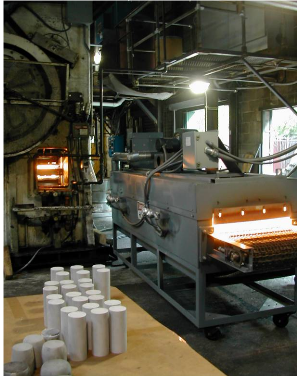
Fig. 4.35. Continuous-belt IR heating furnace installed at Queen City Forging Company, Cincinnati, Ohio.
