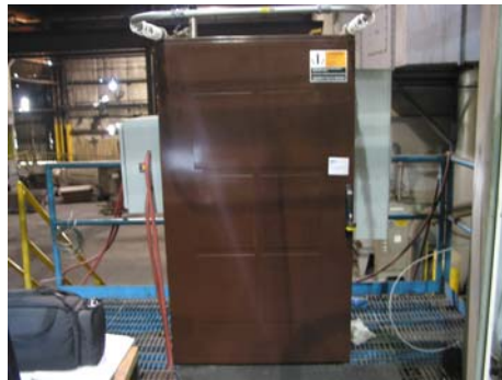
Figure 22 - Instrument Cabinet Located on the Mezzanine
