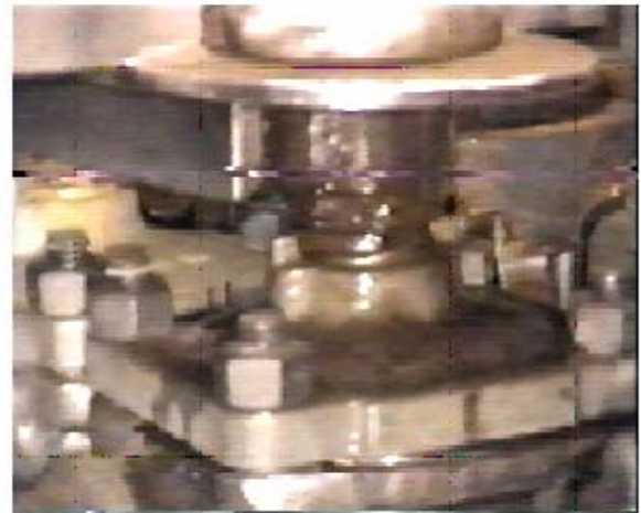
Figure 14: Photographs of Transfer Valve Packing Leak
