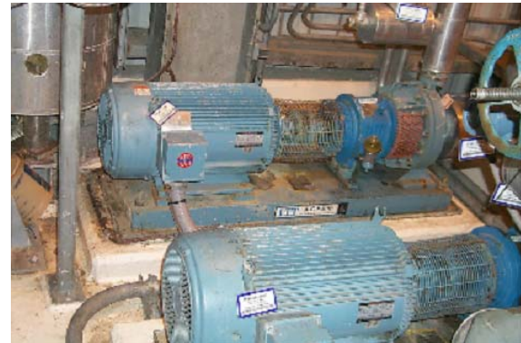
Figure 4: Flush Water Pumps
