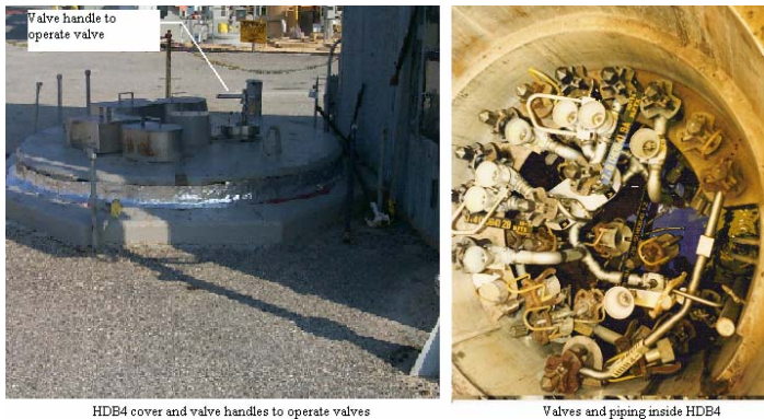
HDB4 cover and valve handles to operate valves
