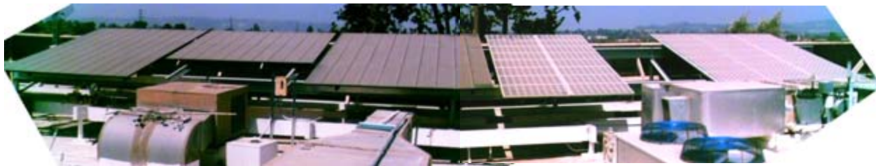
Figure 52. On the left is a 2.88 kW CIS array of 80 ST36 modules. On the right is a 3.0 kW CZ array of 40 ST75 modules.
